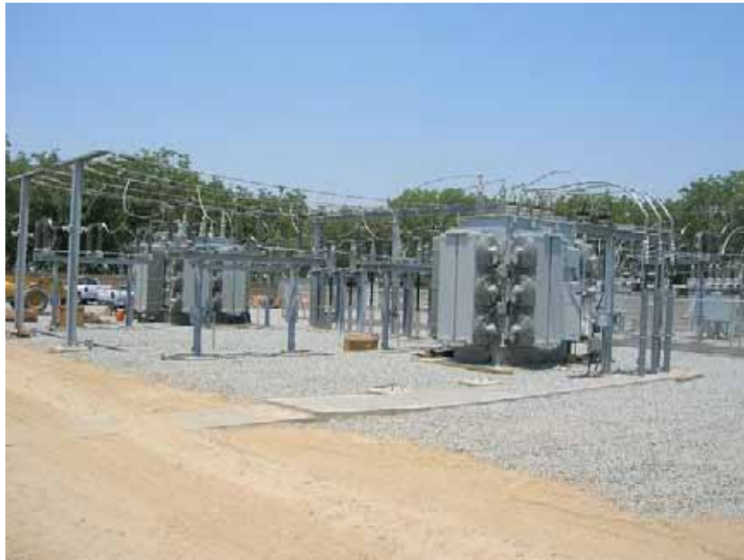
Figure 3: One of the transformers will be activated before the July 4 th holiday and will be tied into the local power grid in order to meet the increased electricity demand expected during the holiday. The remainder of the system will be completed and activated in the near future. The photograph faces northwestward.
