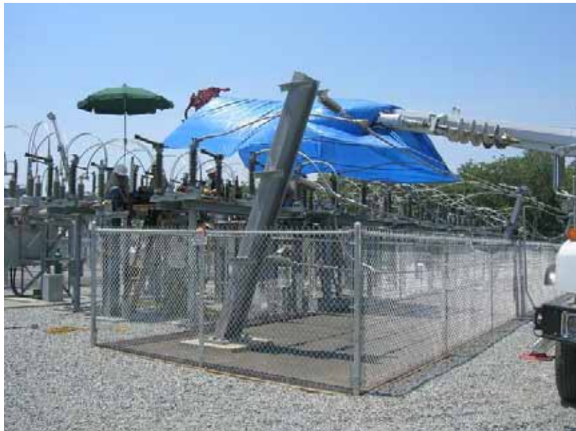
Figure 2: A Southern California Edison crew worked on completion of electrical connections on the incoming 60 KV portion of the sub-station. The photograph faces southwestward.
