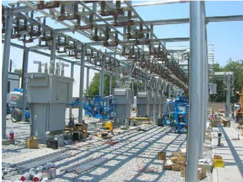
Figure 1: An electrical contractor worked on completion of electrical connections on the outgoing 12 KV portion of the sub-station. The photograph faces westward.
