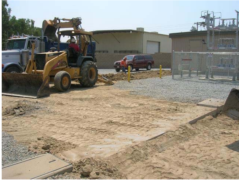
Figure 1: Paved roadways were being constructed within the substation. The photograph faces southeastward, with the MEER building in the background.
