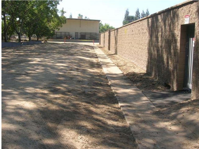
Figure 1: Two shallow V-ditches have been installed to facilitate the drainage from runoff outside the station to retention basins on the north side of the station near the road under construction. The above V-ditch is on the eastern side of the station. The photograph faces southward.
