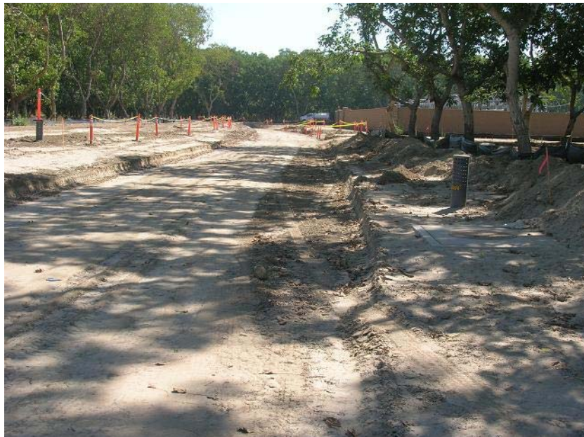
Figure 2: Some work was done on the access road prior to the current work stoppage. The photograph faces eastward.
