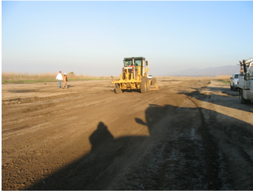
Figure 1: Transport route preparation within MCBCP. Minor grading was required to accommodate the RSGs along the transport route.
