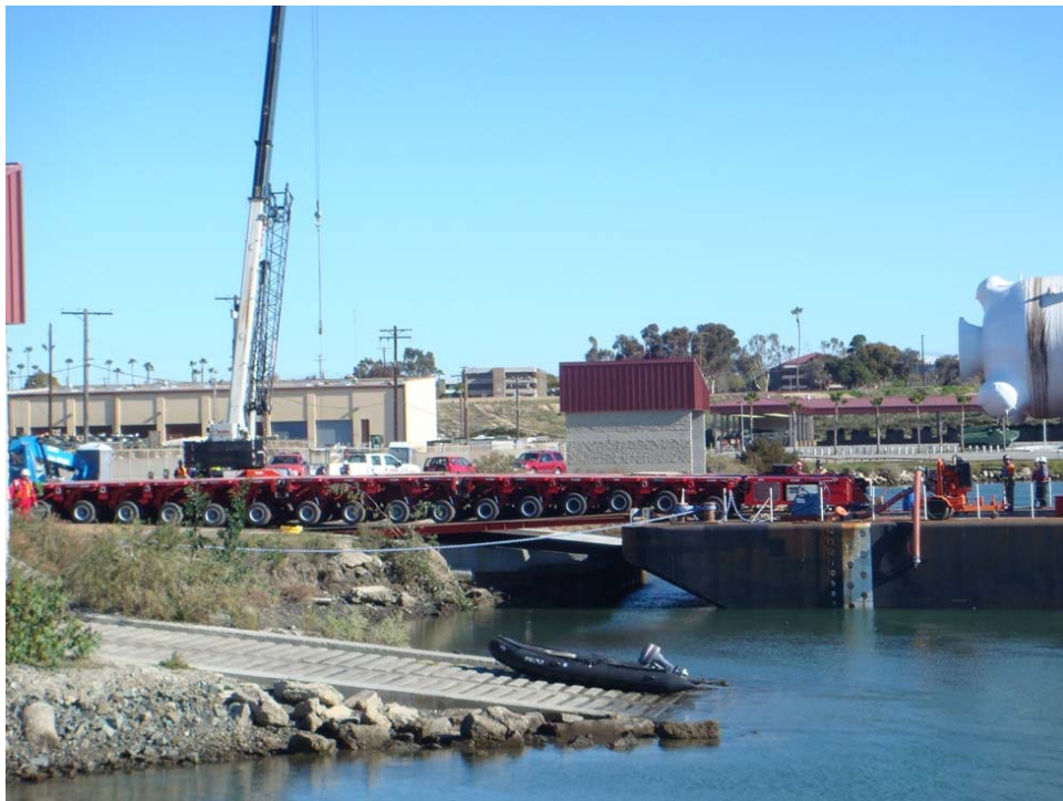
Figure 4: Loading of the Goldhofer onto the barge. The Goldhofer is a series of trailers joined together. During offloading of the first RSG, the Goldhofer experienced axle damage, causing a delay in offloading the second RSG while repairs were made.
