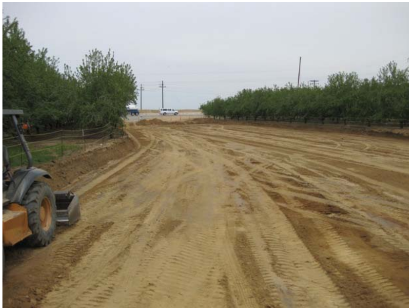
Figure 2: The access road has been excavated except for a section next to Seventh Standard Road (in the distance). This section will be excavated soon in conjunction with coordination with the local roads department, including traffic control. The access road will be filled to grade with imported material. The photograph faces northward.
