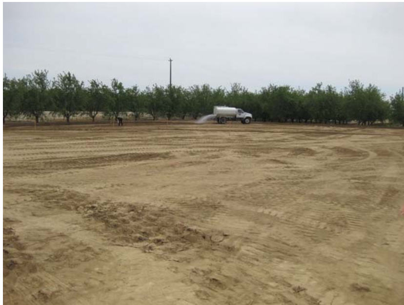
Figure 3: The substation site grading has been mostly completed to sub-grade level. An additional few inches of material will be imported from off site to reach grade. The contractor used a water truck for compaction. So far, dust control has not been necessary because of recent winter rain events and continued cold temperature. The photograph faces southeastward.
