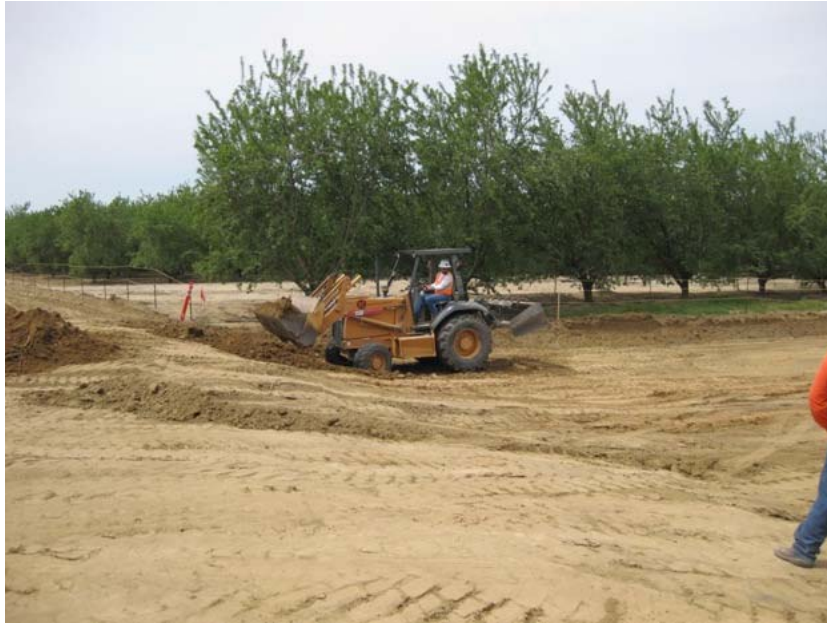
Figure 1: The access road (on the left) has been mostly excavated. The access road will be filled to grade with imported material, and then paved to a sixteen foot width. The photograph faces westward.
