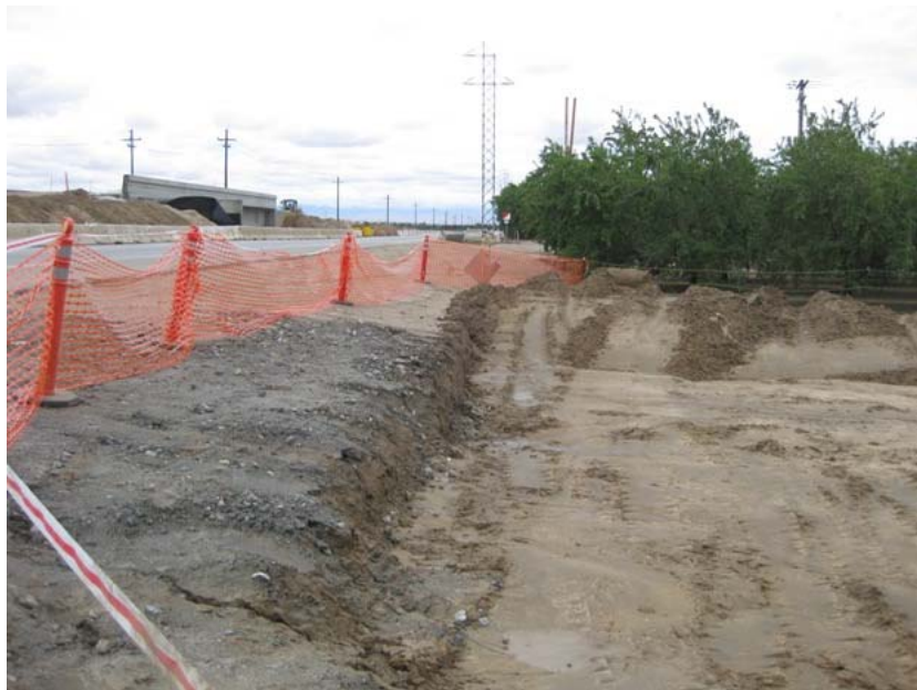
Figure 2: The permit for the construction of the entrance to the access road has been obtained from the City of Bakersfield. The construction will be completed as soon as soil conditions have dried sufficiently. The photograph faces eastward.
