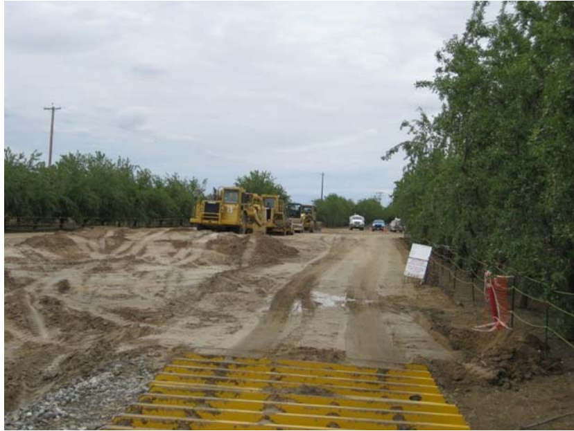
Figure 1: The access road has been excavated. Fill and paving will be conducted after the soil dries out from recent rain events. The shaker plate (see foreground) helps to prevent transportation of dirt onto Seventh Standard Road. The photograph faces southward.
