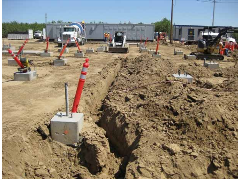
Figure 1: Construction of structure foundations, below-ground conduit trenches, and the ground grid system continued during the subject period. The concrete pad for the transformer was placed (see concrete truck in front of the electrical controls enclosure in the distance). The photograph faces northward.
