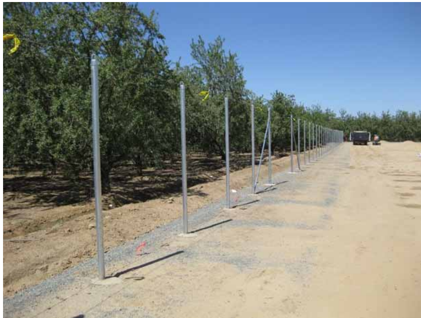
Figure 3: Work on the perimeter chain link fencing continued during the subject period. While under construction the fence was fitted with temporary supporting wiring between the poles. The wires were festooned with yellow flagging to prevent bird collision events. The photograph faces southwestward.
