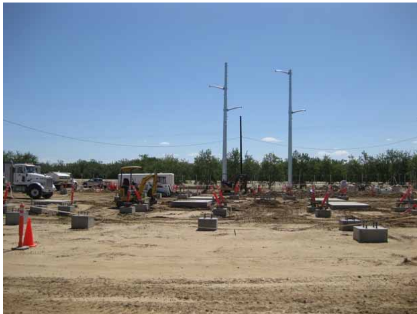
Figure 2: The tubular steel poles were installed near the eastern edge of the site. The photograph faces eastward.
