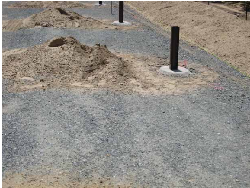
Figure 4: A concrete paneled wall will be placed along the perimeter of the west edge of the substation site in anticipation of future home development in that area. Supports for the concrete wall paneling have been placed. The wall panels are scheduled to arrive in a few weeks.
