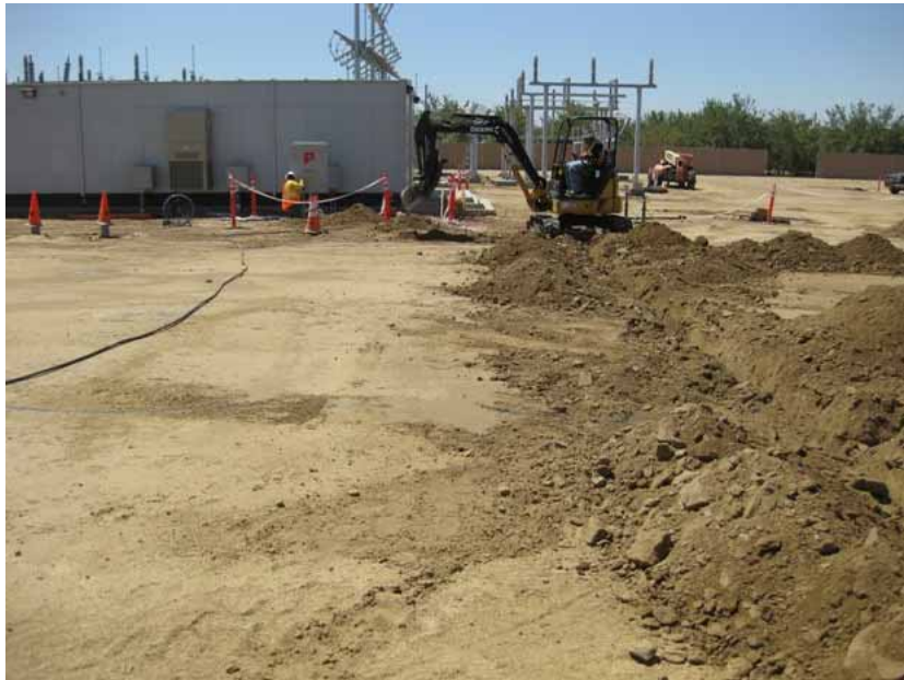
Figure 2: Below-ground conduit trenches were being excavated leading to the electrical controls enclosure in the middle distance. The photograph faces southward.
