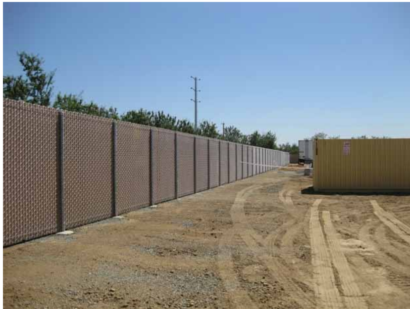
Figure 3: Work on the perimeter chain link fencing has been mostly completed. The eight-foot high chain link fencing is being installed on both sides of the access road and along the south, north and east boundaries of the substation. The photograph shows the north side fence, and faces northeastward.
