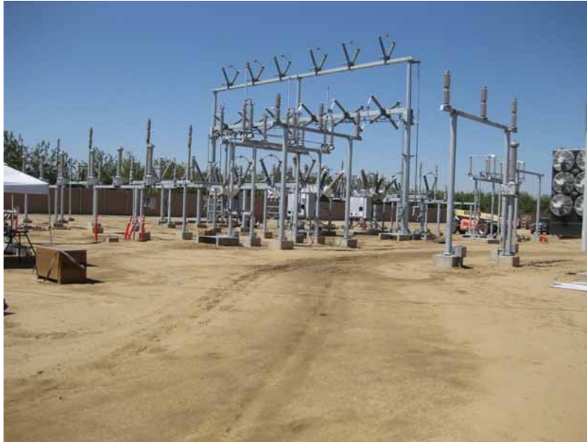
Figure 1: During the subject period, erection of structures continued. The photograph faces southwestward.
