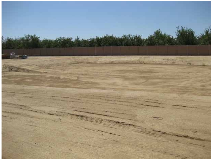
Figure 5: The contouring for the retention basin has been started in the western portion of the site. Some of the remainder of the western portion of the site is being utilized for vehicle and equipment parking, and for materials storage. This section may be used for future substation expansion. The photograph faces southeastward.
