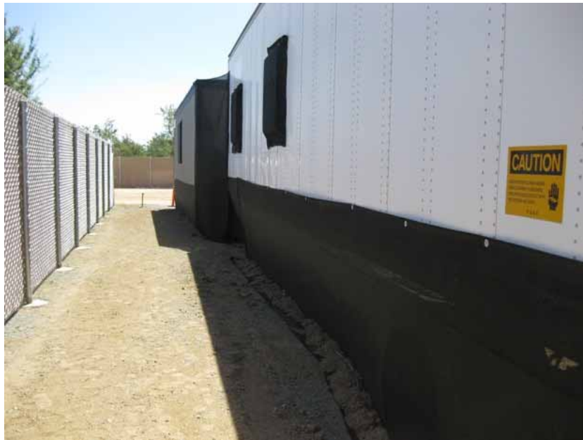
Figure 7: Black netting has been placed around the opening under trailers to discourage nesting by birds such as the black phoebe. The photograph was taken near the northern perimeter fence, and faces eastward towards the access road in the distance.
