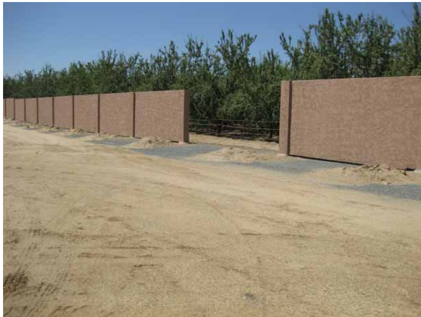
Figure 4: A concrete paneled wall was placed along the perimeter of the west edge of the substation site in anticipation of future home development in that area. An access gate will be placed in the middle of the wall. The photograph faces southwestward.
