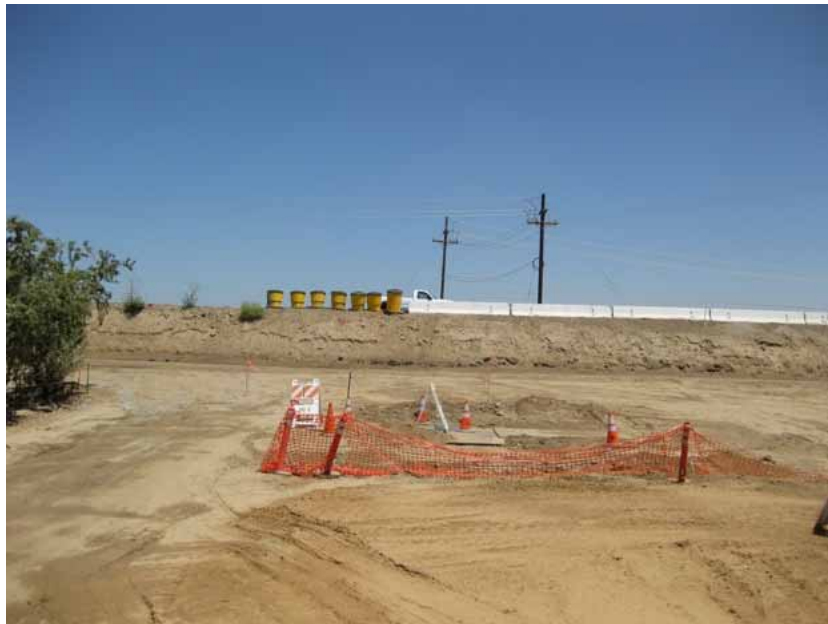
Figure 6: Final grading of the access road (in the foreground) is awaiting the completion of the rebuilding work on Seventh Standard Road at the entrance to the access road. The former two-lane roadway has been removed, and will be replaced with two new eastbound lanes. The new westbound lanes have been completed (beyond the K-rails), and are currently carrying both directions of traffic. The photograph faces northward.
