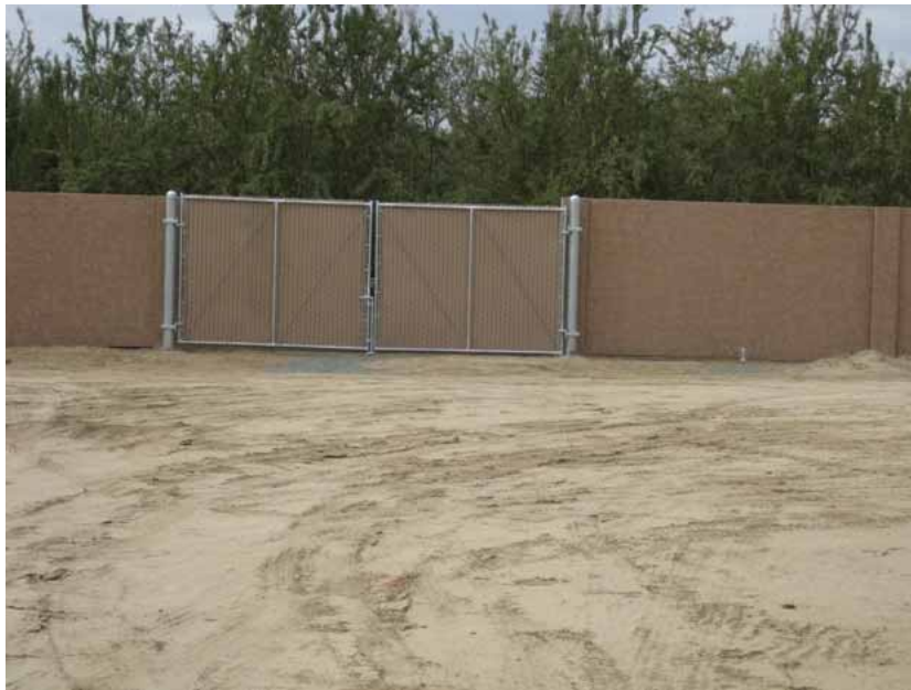
Figure 3: The access gate in the concrete wall along the perimeter of the west edge of the substation site was installed during the subject period. The photograph faces westward.
