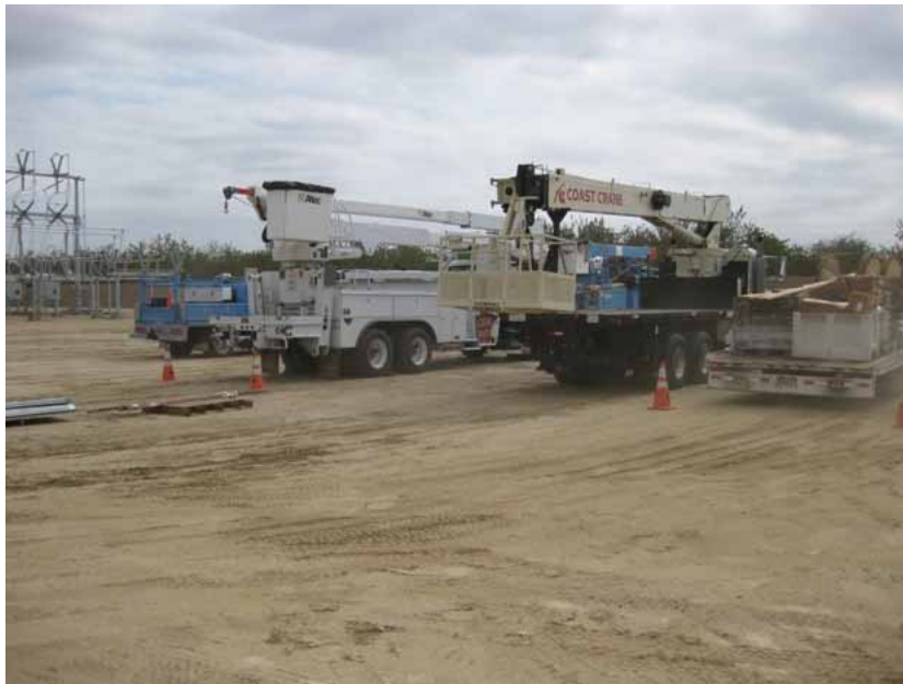
Figure 5: During the subject period, the PG&E line crews working on the installation of the final two tubular steel poles and on the stringing of conductor into the substation used the western portion of the substation site for staging. The photograph faces southeastward.
