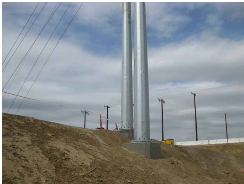
Figure 2: The final two tubular steel towers were installed and conductor was strung. They are adjacent to highway construction on Seventh Standard Road.
