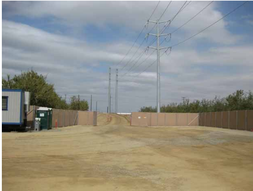
Figure 1: Final connections with outside lines, including the installation of the final two tubular steel poles (in the distance), were completed by PG&E crews during the subject period. Also, the fencing was constructed across the entrance to the substation. The photograph was taken in the eastern portion of the substation site, and faces northward toward the access road.
