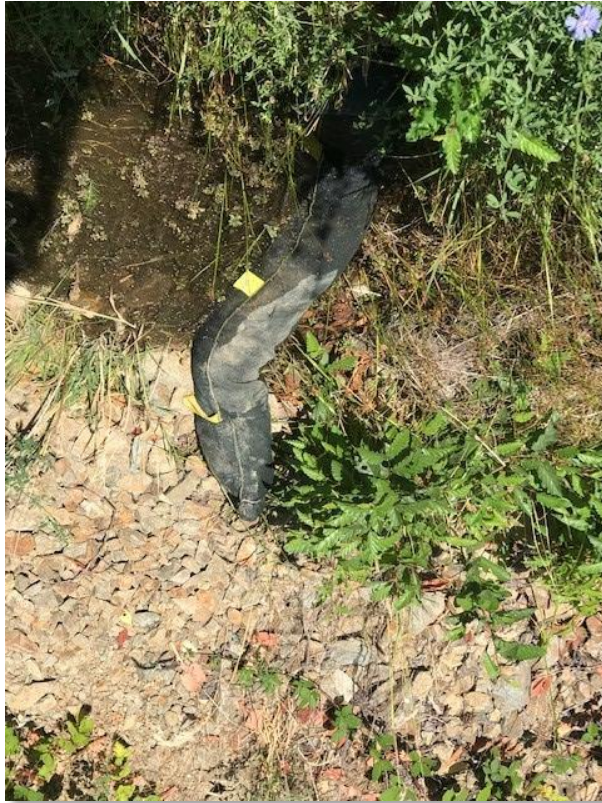
Figure 9. Fiber roll in place for sediment control in drainage at MP 28.75 (July 24, 2019)
