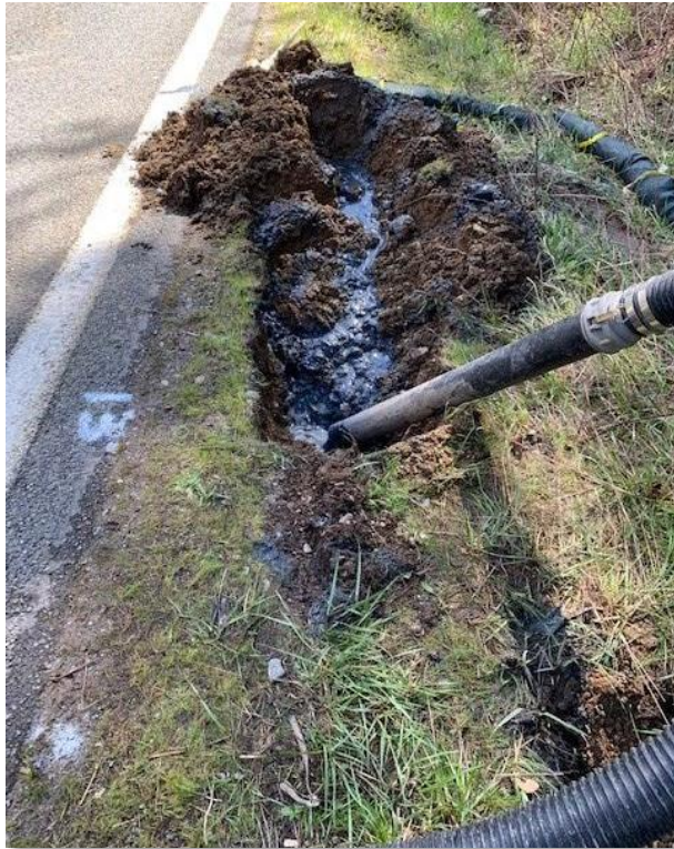
Figure 6. Frac-out at MP 31.51 into a culvert outfall (March 28, 2019)
