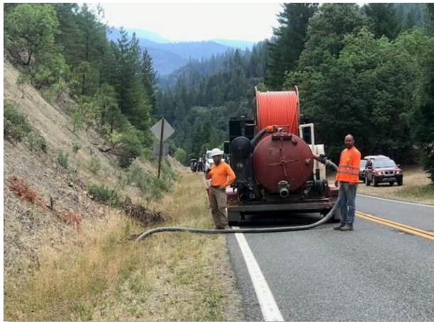
Figure 8. Vac truck placed in position to clean up frac-out at MP 29.8 (August 28, 2019)
