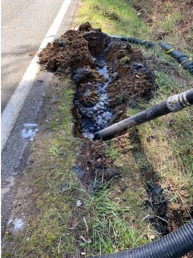
Figure 5 – Frac-out at MP 31.51 – view south, March 28, 2019. Photo courtesy of Siskiyou Telephone.
