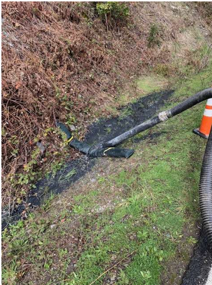
Figure 4 – Frac-out at MP 31.79 – view northwest, March 26, 2019. Photo courtesy of Siskiyou Telephone.
