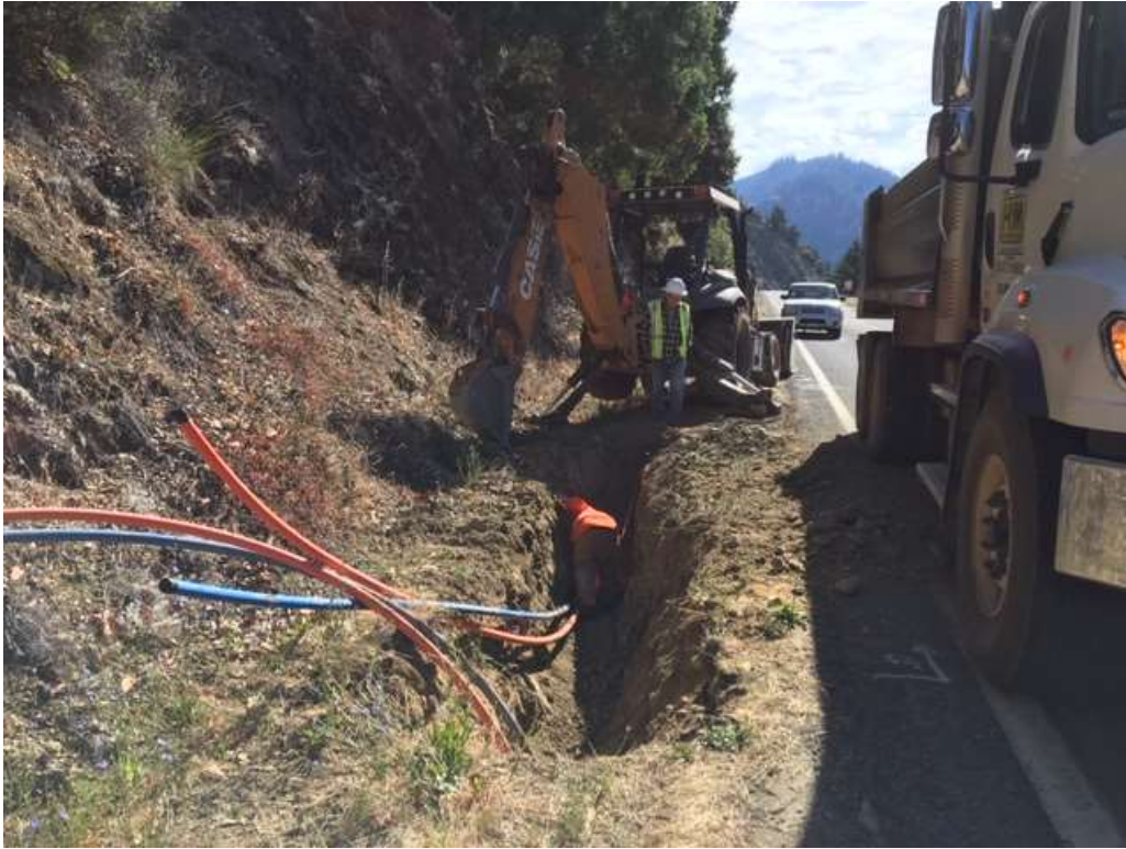
Figure 1 – Crew digging and excavating for tie-in-box at MP 24.04 southwest along Hwy 96 – view north, July 10, 2019.
