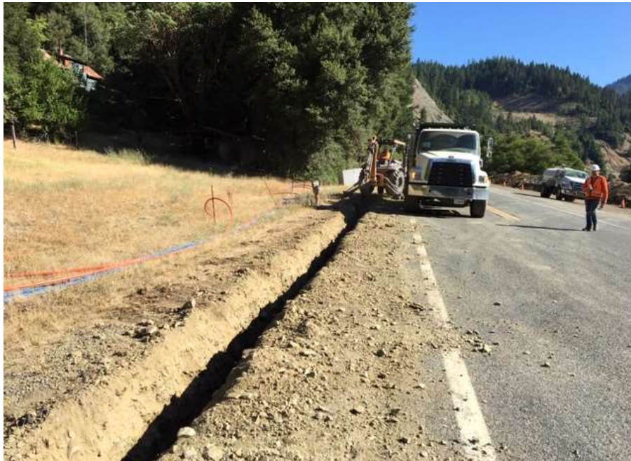
Figure 2 – Crew trenching in conduit at MP 28.5 southwest along Hwy 96 – view north, July 24, 2019.
