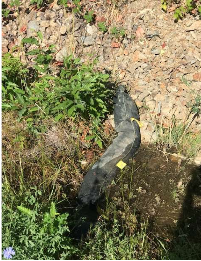
Figure 1 – Fiber roll in place for sediment control in drainage at MP 28.75 - July 24, 2019.
