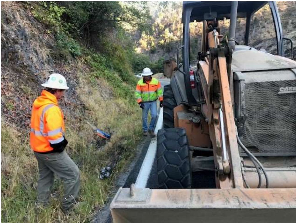
Figure 1 – First crew with drill bit popped out and equipment staged properly in the road at MP 15.94– view north, September 11, 2019.
