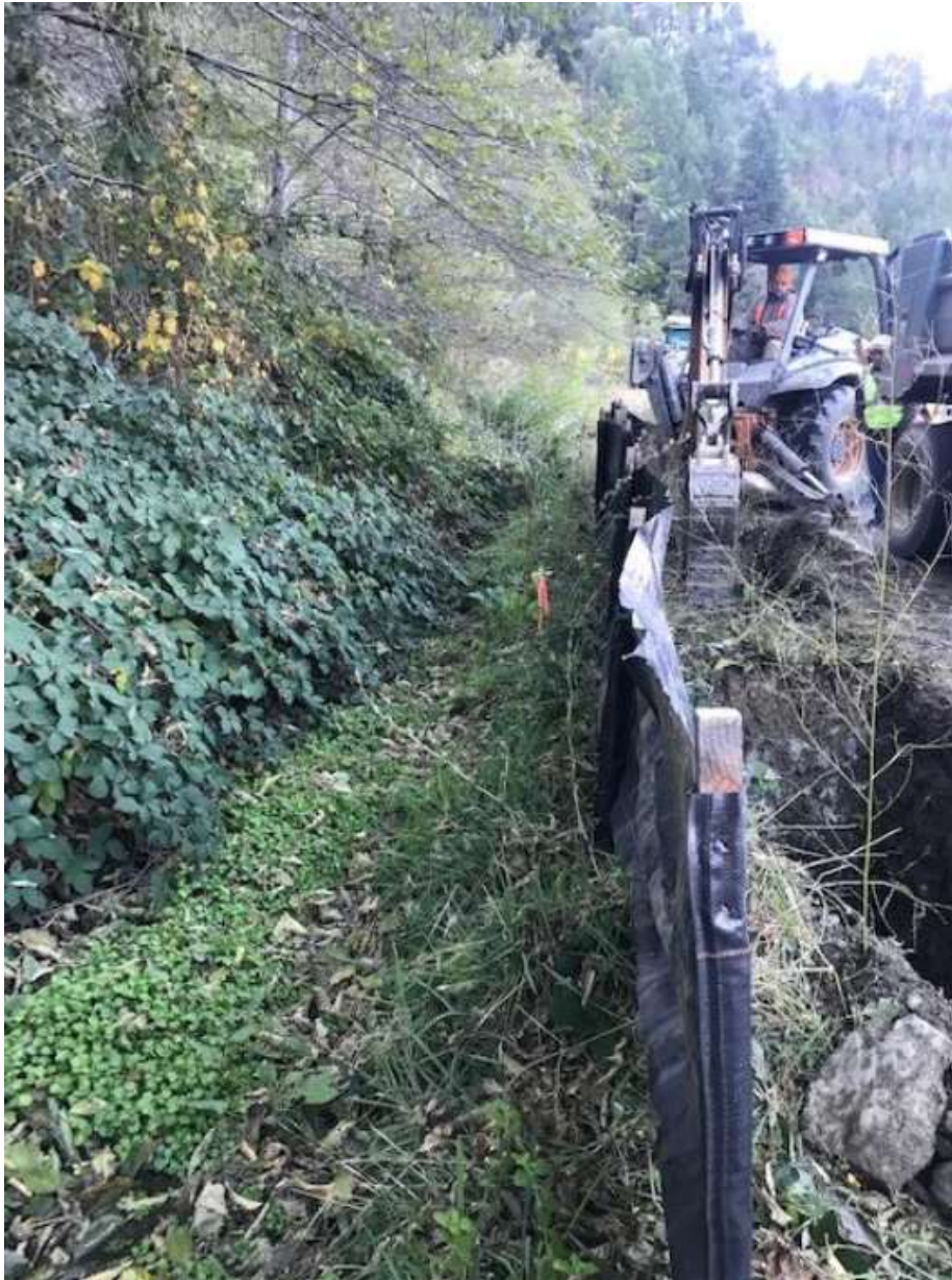
Figure 4 – Silt fence and tie-in work adjacent to sensitive habitat at MP 13.75, October 30, 2019.
