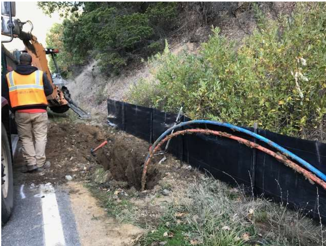
Figure 11 – Crew digging adjacent to sensitive habitat at MP 13.31 with silt fence installed, October 31, 2019
