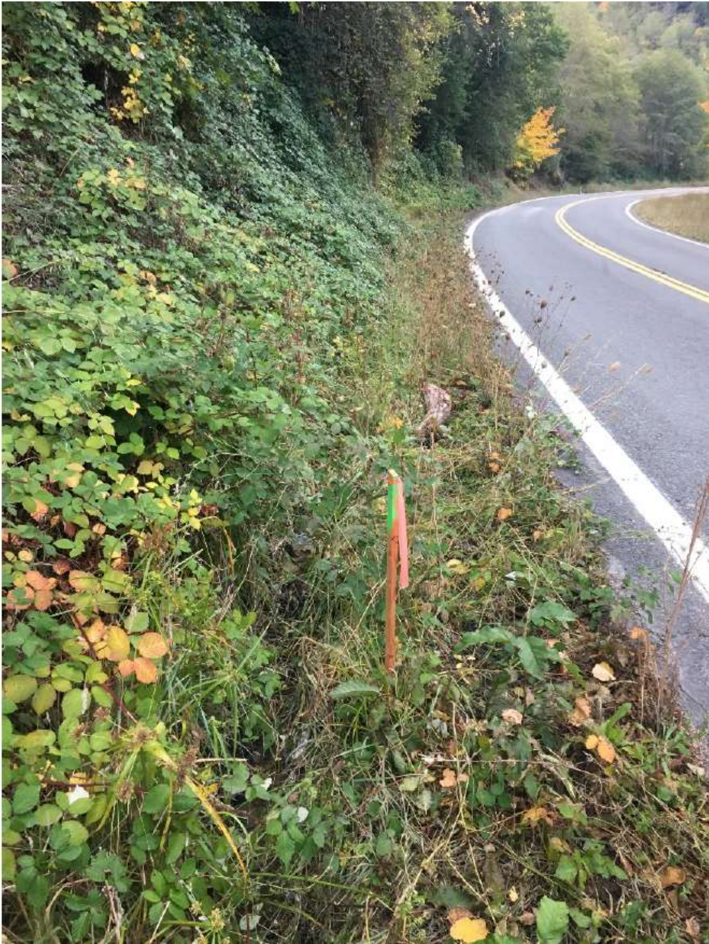
Figure 2 – Cleaned up location within sensitive habitat where nominal frac-out of bore mud occurred at MP 13.90, October 24, 2019.
