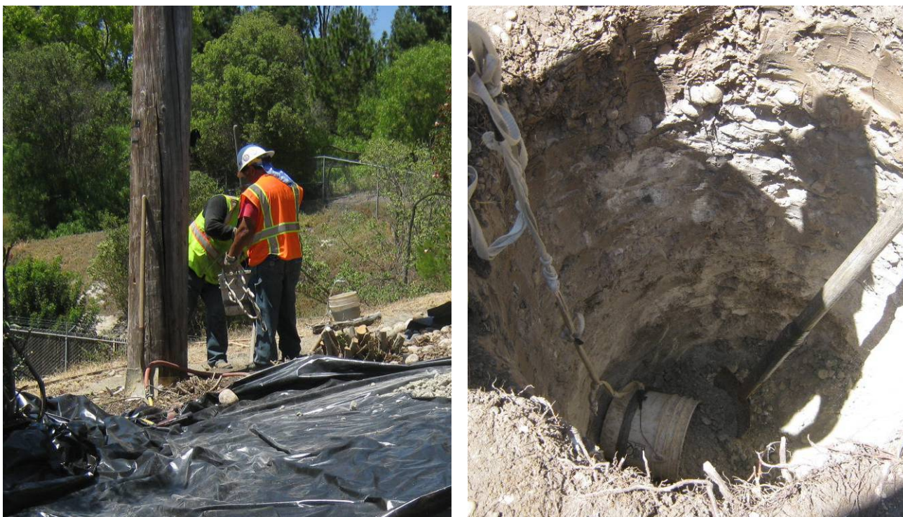
Figure 14. Hand-digging for pole replacement at location Z775593 along the 69 kV TL693, west of Link 5 and south of Tierrasanta Boulevard. Fossils were discovered at a depth of 8 feet below the surface in fine-grained sandstones of the Friars Formation. Bulk sedimentary matrix was screenwashed and heavy liquid separation processed. This locality (SDNHM Locality 6302) produced over 100 specimens of Eocene-age, small mammal teeth.
