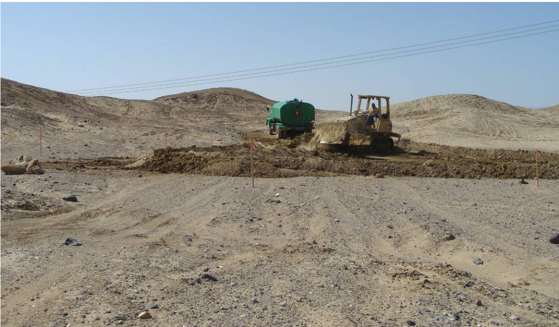
Figure 3. Grading of access road for EP322 in Recent colluvium overlying strata of the Arroyo Diablo Formation; Link 1.
