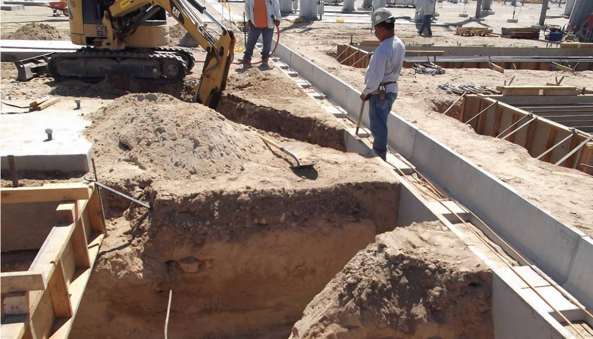
Figure 2. Equipment footing excavation by PAR Electric within the Imperial Valley Substation exposing Lake Cahuilla strata; Link 1.
