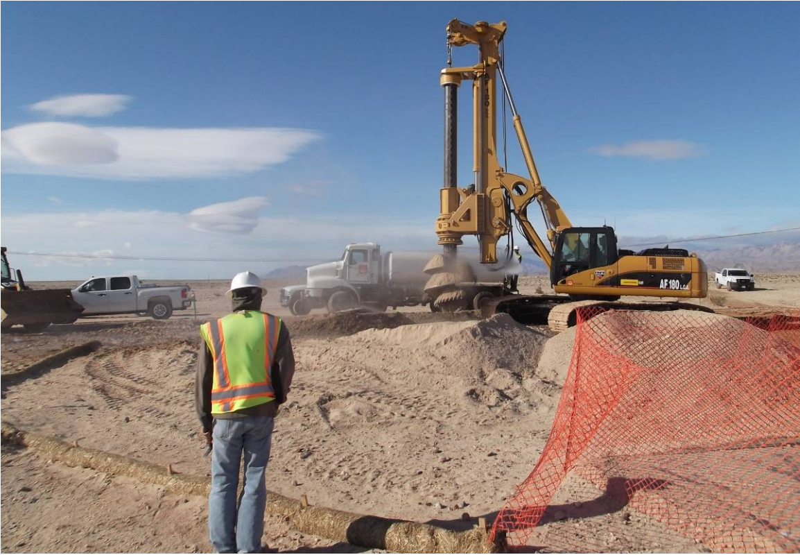
Figure 5. Drilling for tower footings at EP 341. Older alluvium at the ground surface overlies Palm Spring Group sandstones, siltstones, and mudstones at depth; Link 1.
