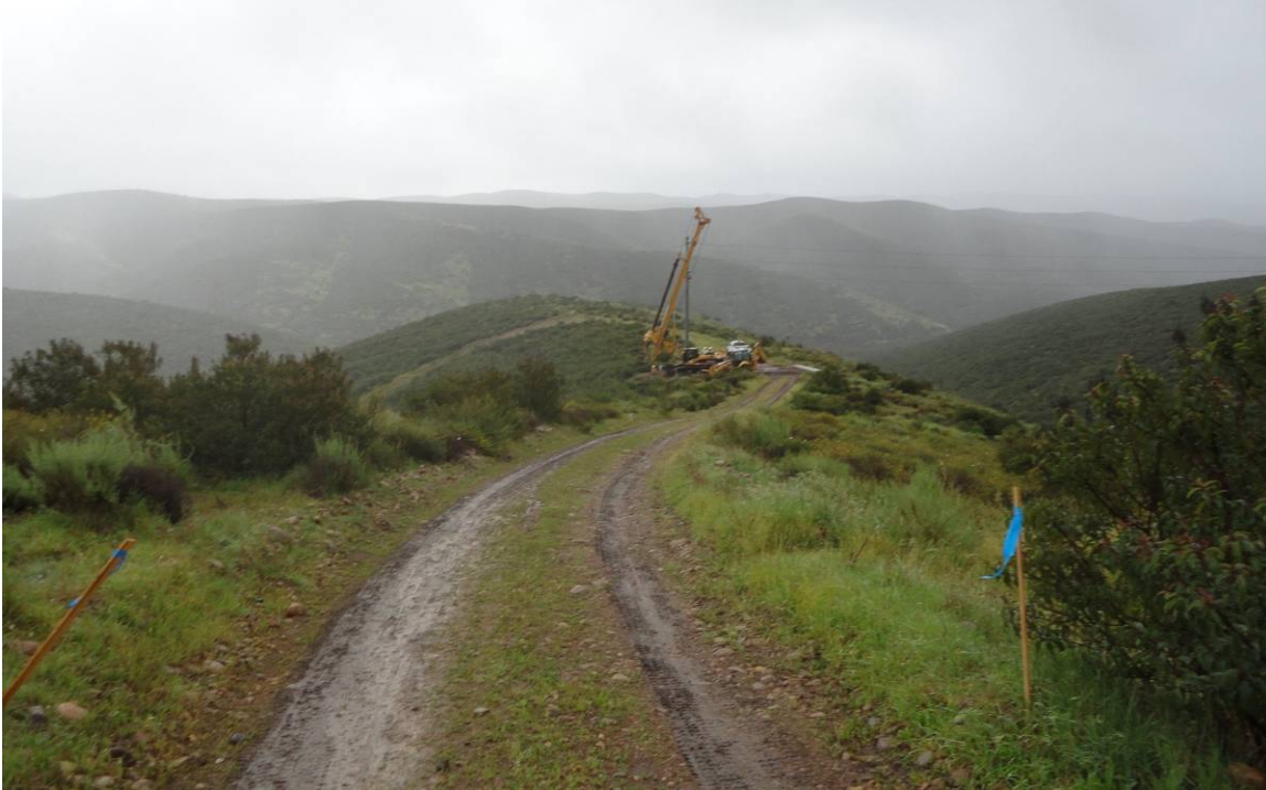
Figure 6. Drilling for tower footings at CP17 in Eocene strata of the Stadium Conglomerate; Link 5.
