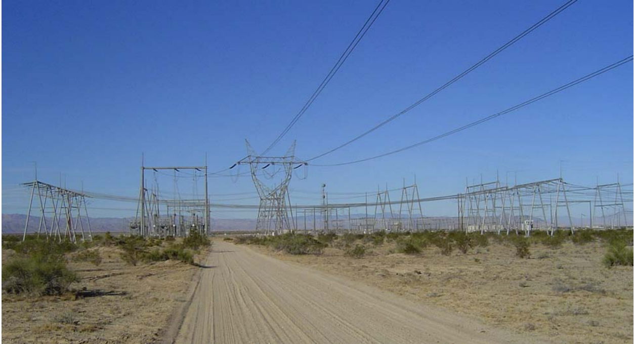
Imperial Valley Substation
