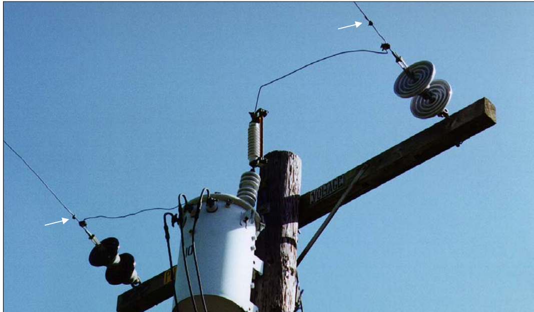
Figure 3-38 Idle Split Bolt Connectors
