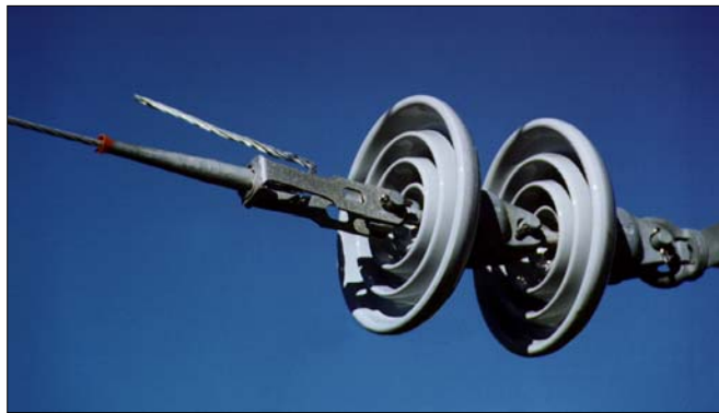
Figure 3-45 Automatic Deadends with Suspension Insulators
