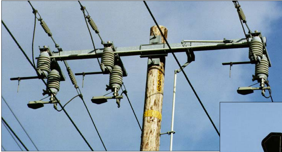
Figure 3-16 600 Amp Underarm Sidebreak Switch (open position)
