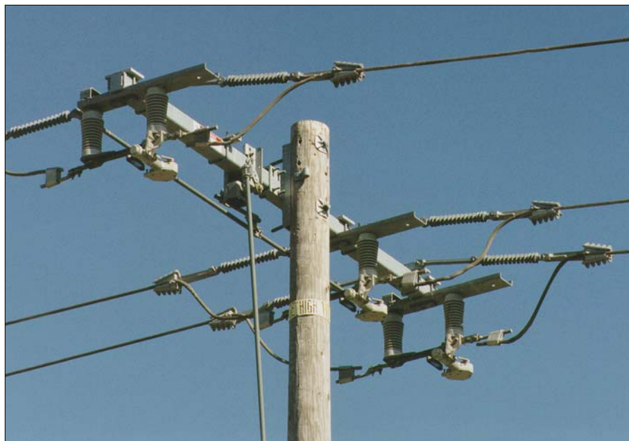
Figure 3-18 S&C Underarm Side-Break Switch (closed position)
