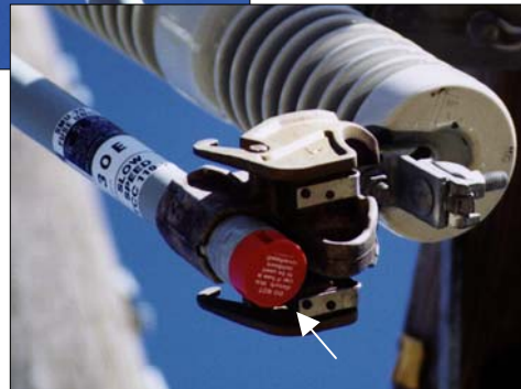
Figure 3-9 SMU-20 Fuse - Detail
