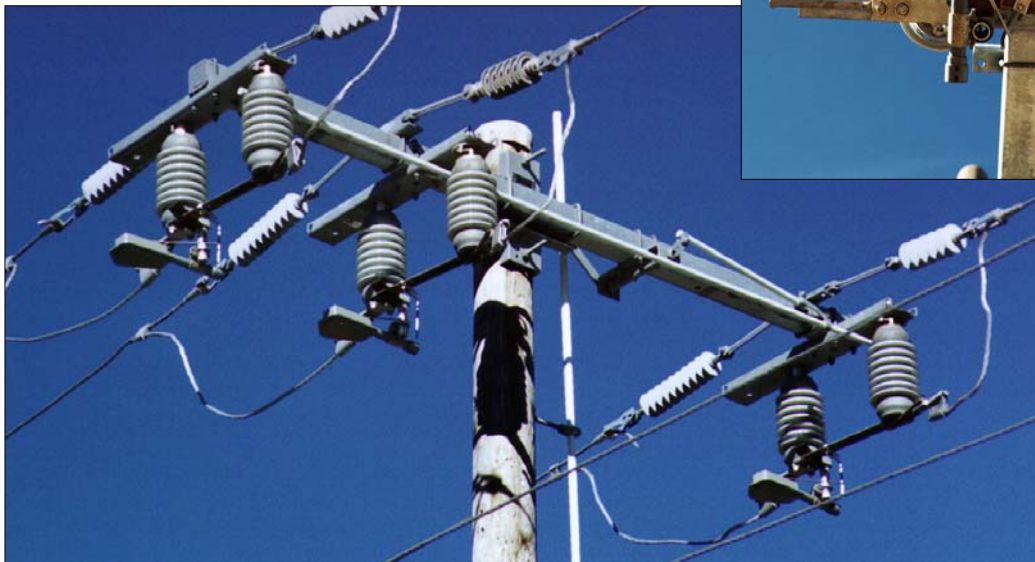
Figure 3-17 600 Amp Underarm Sidebreak Switch (closed position)
