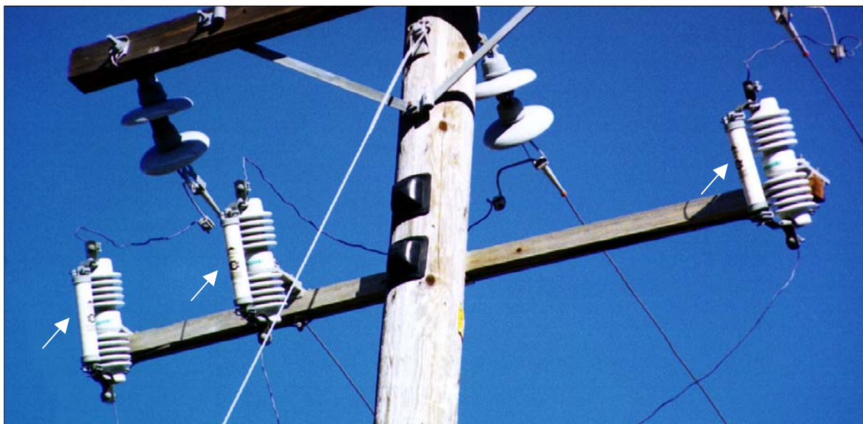
Figure 3-3 Arm Mounted Cutout with Non-Expulsion Fuses
