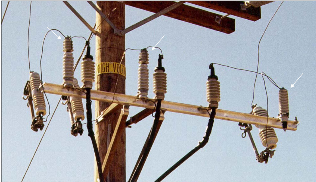
Figure 2-16 Arm Mounted Lightning Arrester (with Cable Riser and Universal Fuses)
