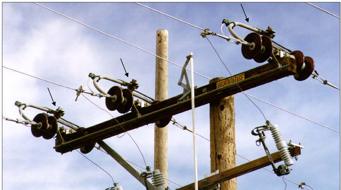
Figure 3-15 600 Amp KPF Air Switch, Crossarm Construction (closed position) Without Arcing Horns or Snuffers
