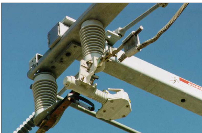
Figure 3-19 S&C Underarm Side-Break Switch (closed position)
