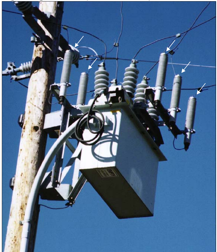
Figure 2-17 Lightning Arrester (with Recloser)
