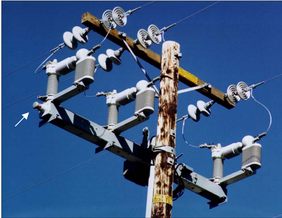
Figure 3-22 S&C Scada-Mate Switch
