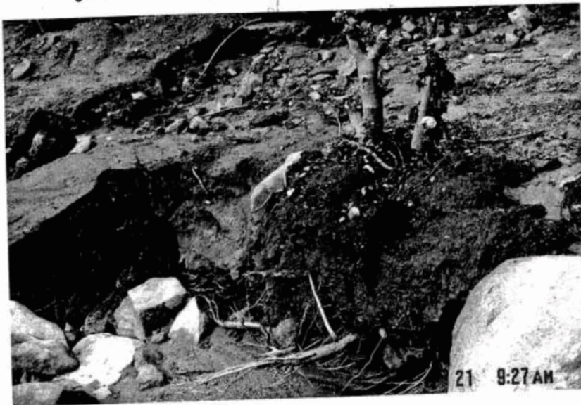
Plants washed away from attempt to culvert. Dirt onto our lower property from SDB&E
