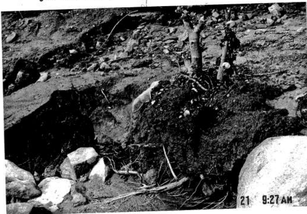
Plants washed away from attempts to culvert. DIRT onto our lower property from SDE&E
