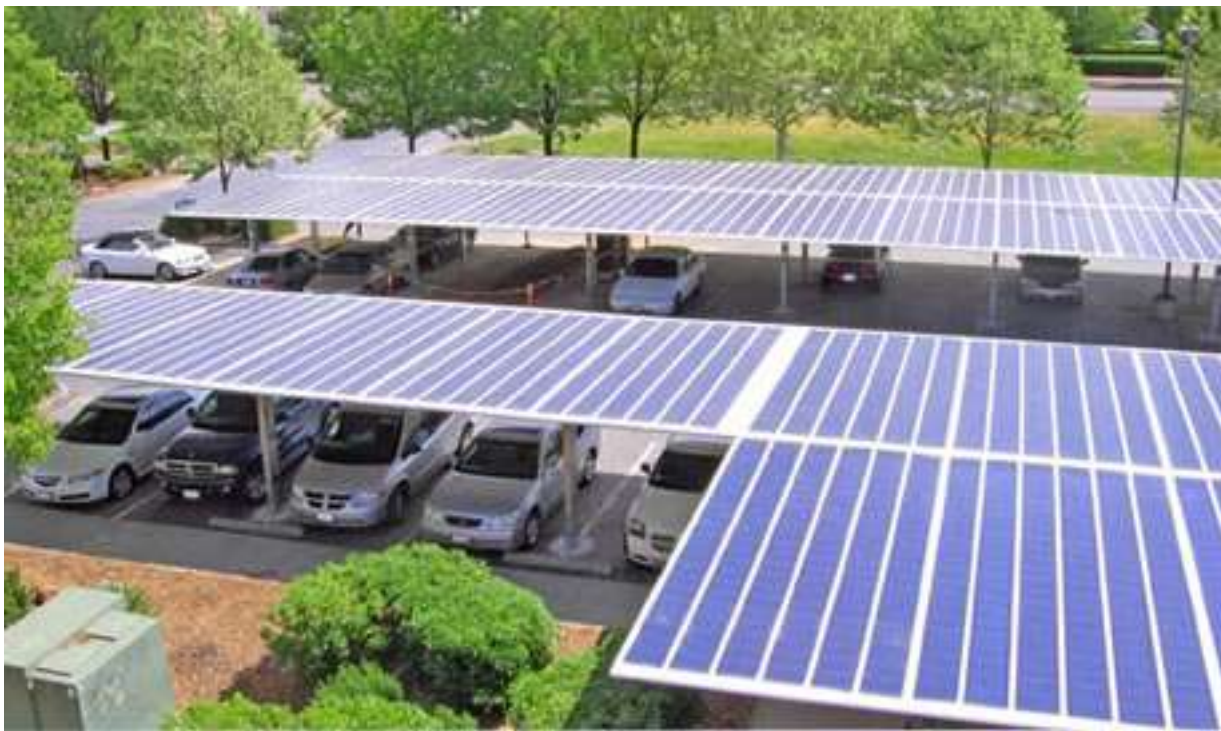
153 kilowatt from a solar carport in Vacaville California
