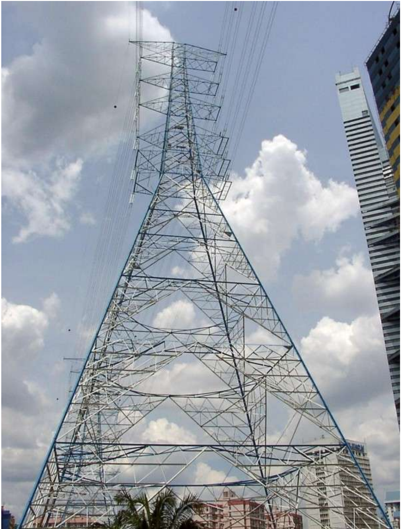
24 cable, high-capacity pylon in Kuala Lumpur Malaysia, 689 foot height
