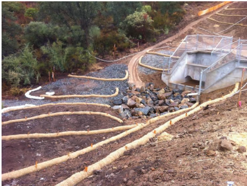
Figure 10: BMPs at northern dissipater, post-rain event. (Link 3)
