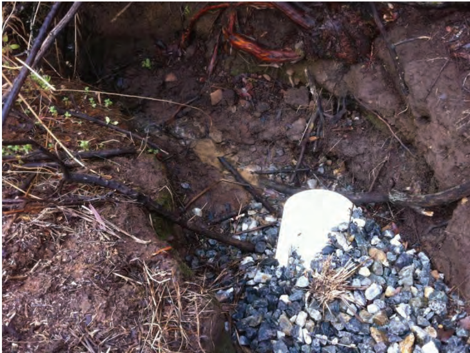
Figure 11: Water seen draining from the northern dissipater. (Link 3)
