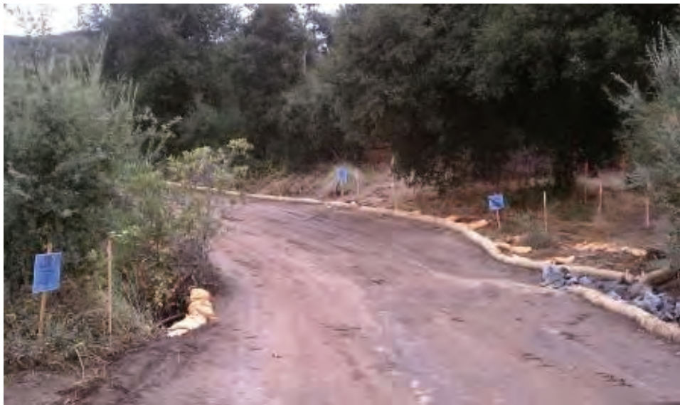
Figure 6: Stormwater BMPs along the access road to CP98, CP99-2 and CP100-1. (Link 2)
