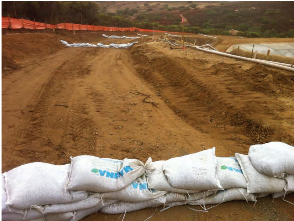
Figure 7: Gravel bags placed along unfinished access road. (Link 3)
