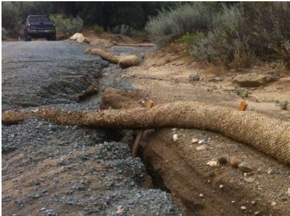
Figure 2: Failed BMP along La Posta Road. (Link 2)
