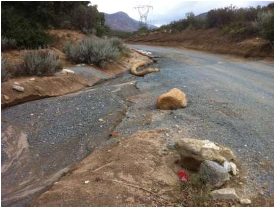
Figure 3: Failed BMP along La Posta Road. (Link 2)
