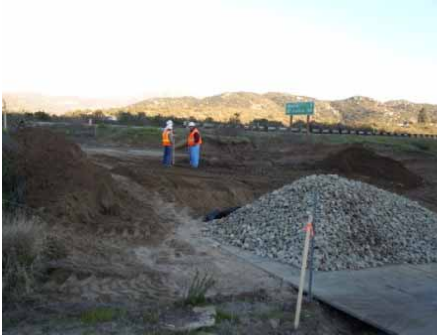
Figure 1: Vegetation clearing on the south side of Interstate 8 at the jack and bore, Link 4.
