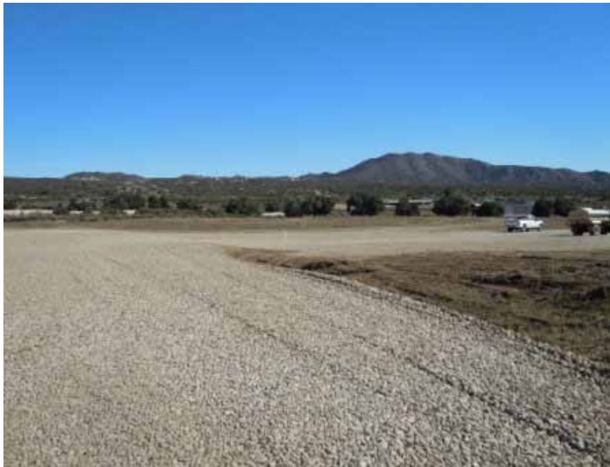
Figure 4: Road base delivered and spread for the parking and helicopter area at the Rough Acres Construction Yard.
