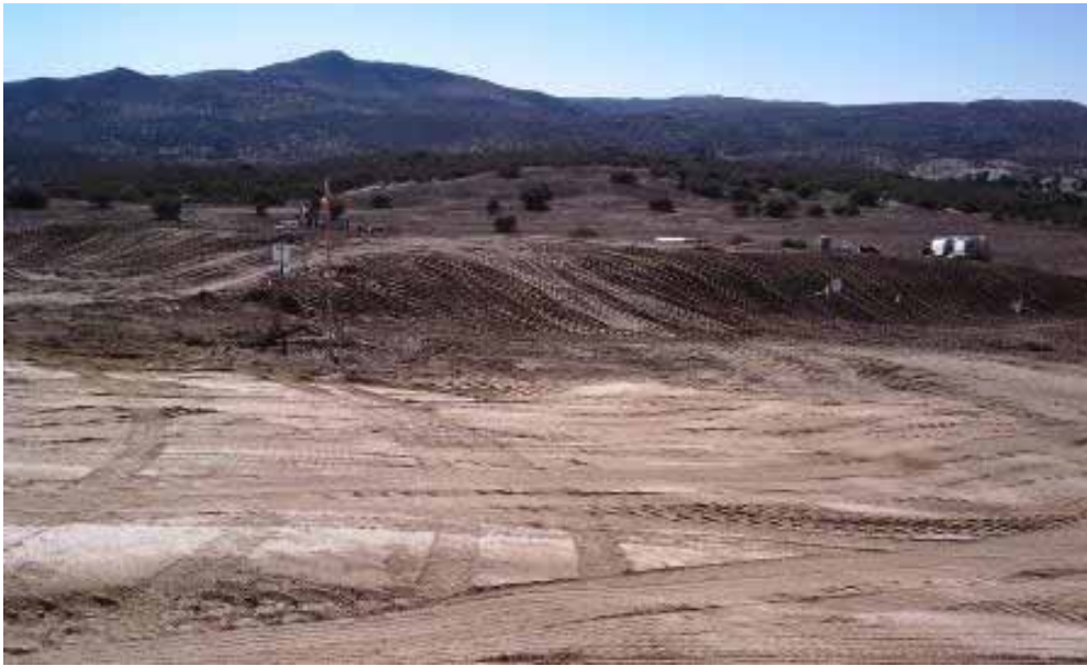
Figure 11: Stockpiling of topsoil on USFS land at Thing Valley Construction Yard. ( Link 2 )
