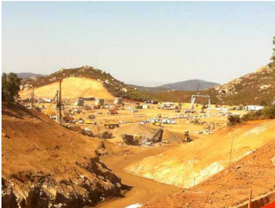
Figure 7: View of Suncrest Substation pad. (Link 3)
