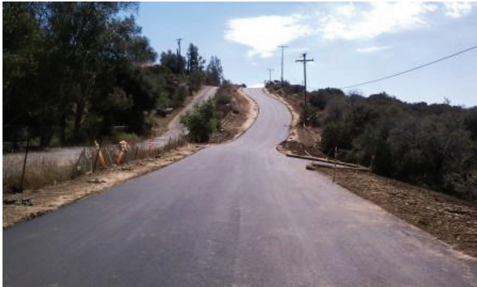
Figure 7: Hydromulching was installed on the sides of the newly paved access road to CP95-1, CP96-1, and CP98. (Link 2)
