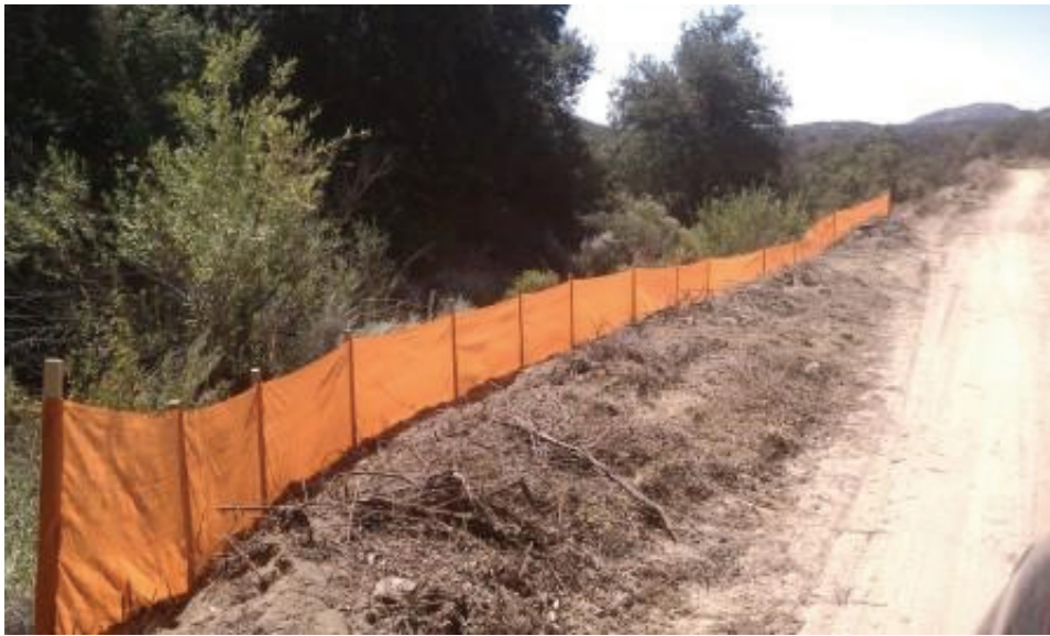
Figure 6: Silt fence adjacent to a creek on La Posta Road. (Link 2)
