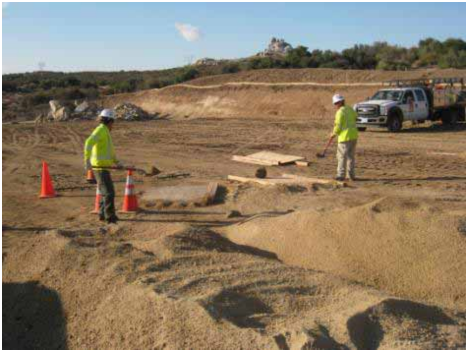
Figure 1: Crews covering foundations holes per the Mitigation Measures at EP219 pull site. (Link 1)
