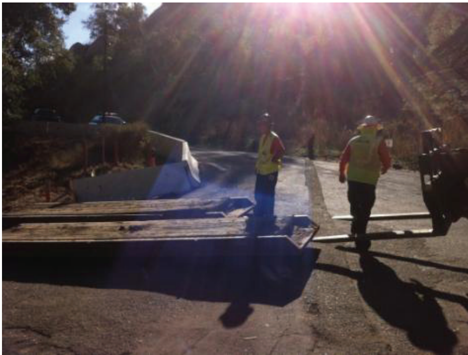
Figure 11: Temporary bridge being set over water line at CP70-3 access road. (Link 5)
