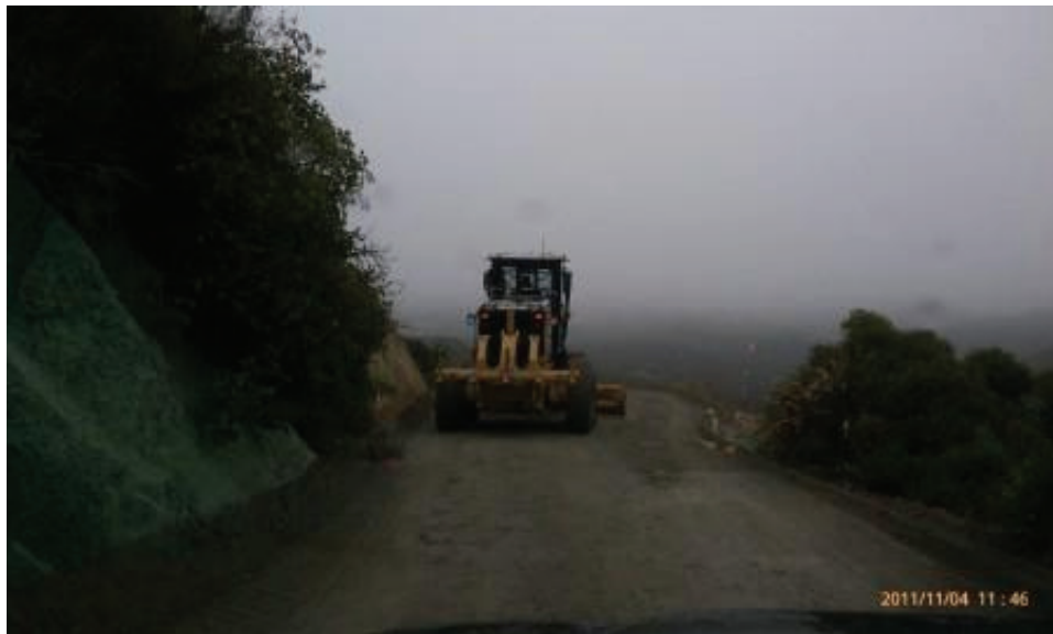
Figure 6: Grading along upper portions of La Posta Road during a rain event. (Link 2)
