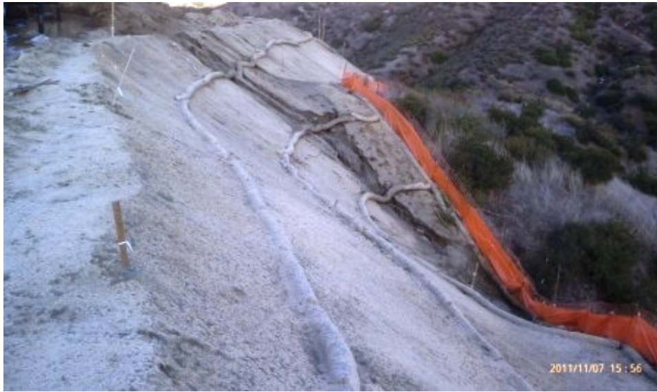
Figure 7: Slope cuts caused by runoff from Slay Property riser pole work site. (Link 4)
