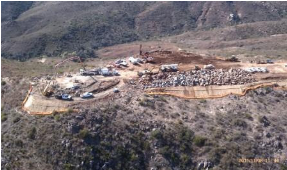
Figure 1: Helicopter view of concrete pouring at EP42 tower site and pull site. (Link 2)
