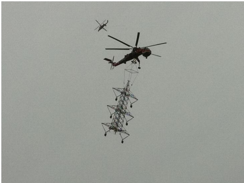
Figure 4: Aircrane and KMAX during tower assembly activities in El Monte Valley. (Link 5)
