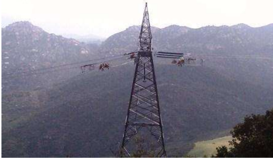
Figure 7: Clipping at Tower EP10. (Link 2)
