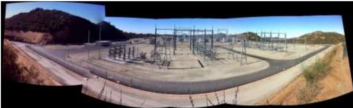
Figure 4: Panoramic view of Suncrest Substation. (Link 3)
