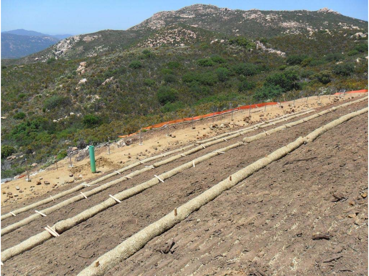
Slope stabilization and erosion control at the southwest corner of Suncrest Substation. Photo courtesy of Mark Meridith.
