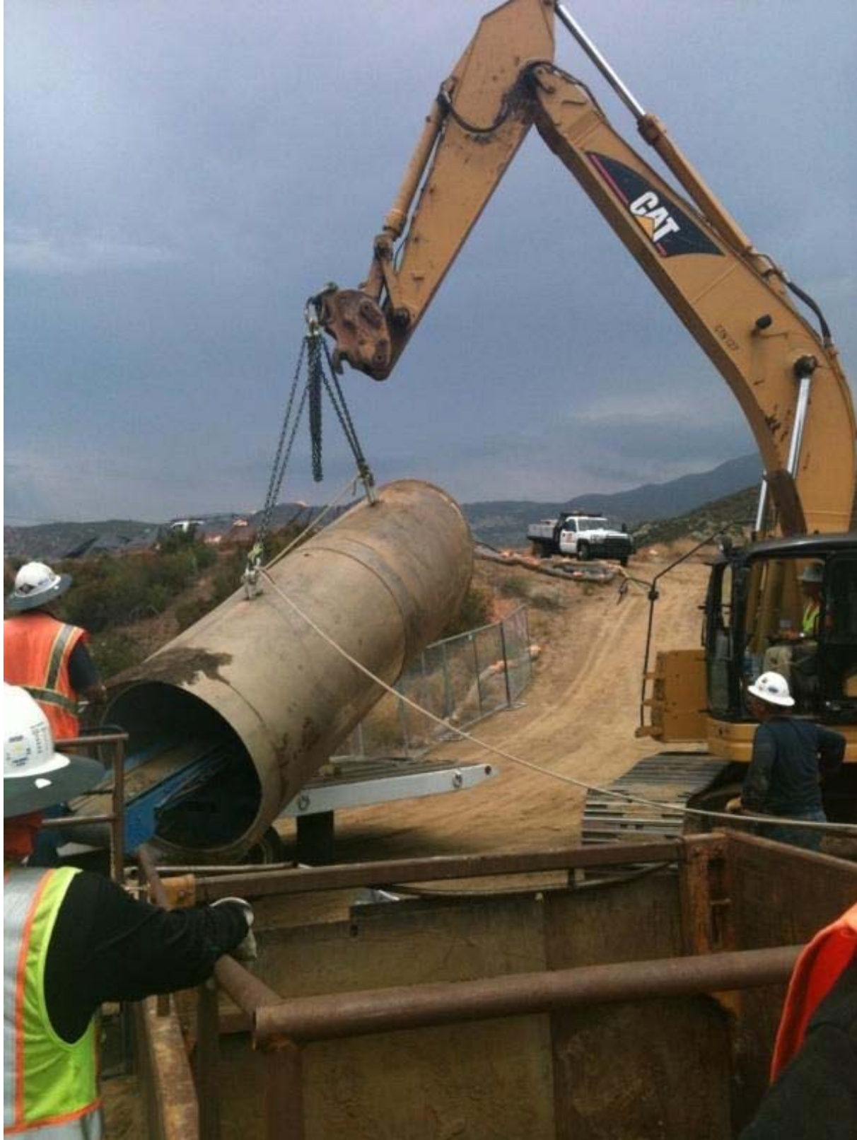
The bore head after removal from the CalTrans bore pit (North of Highway 8). Photo courtesy of Jeff Smith.
