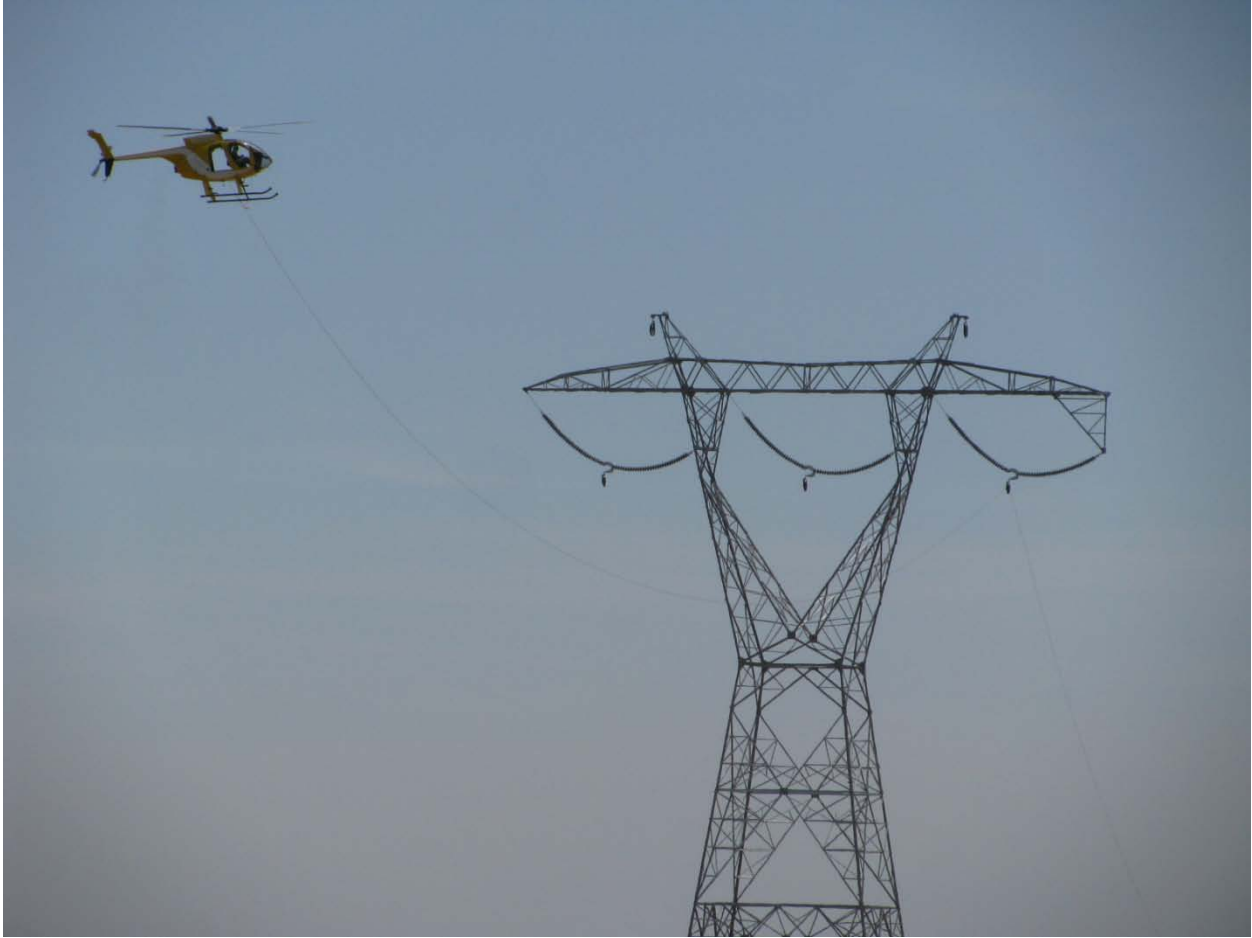
Wire stringing operations for the span between EP330 and EP338. Photo courtesy of Erik Strods.
