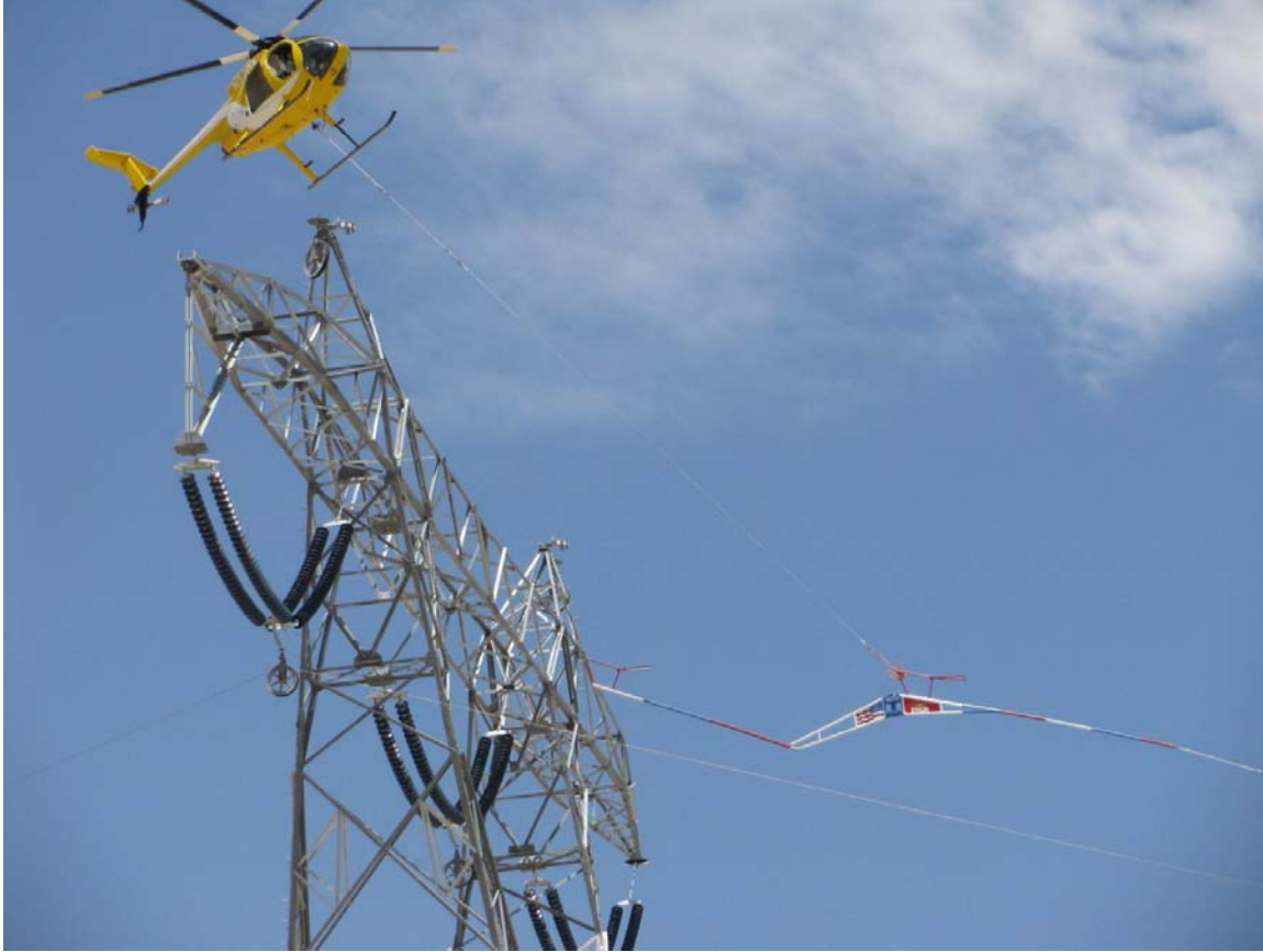
Wire stringing operations for the span between EP330 and EP338. Photo courtesy of Erik Strods.
