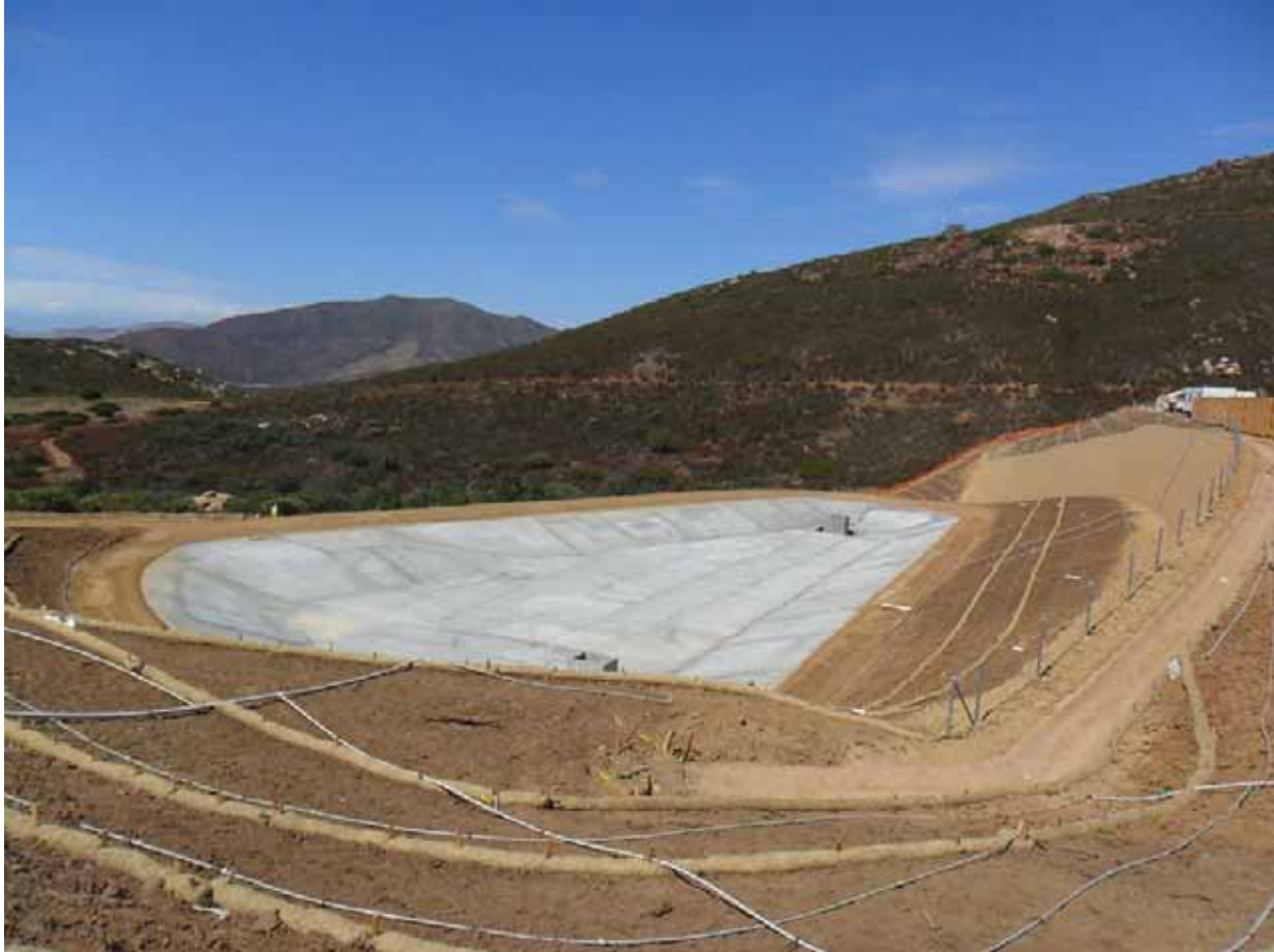
Final grade north sediment basin at Suncrest Substation. Photo courtesy of Mark Meridith.
