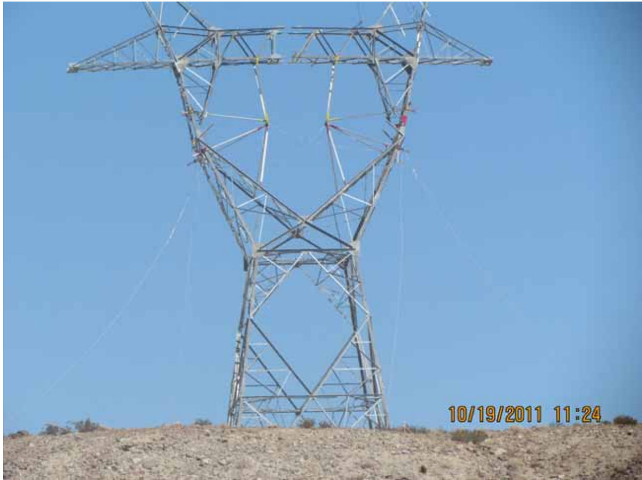
Erecting the 100 th lattice tower at EP290. Photo courtesy of Don Anders.
