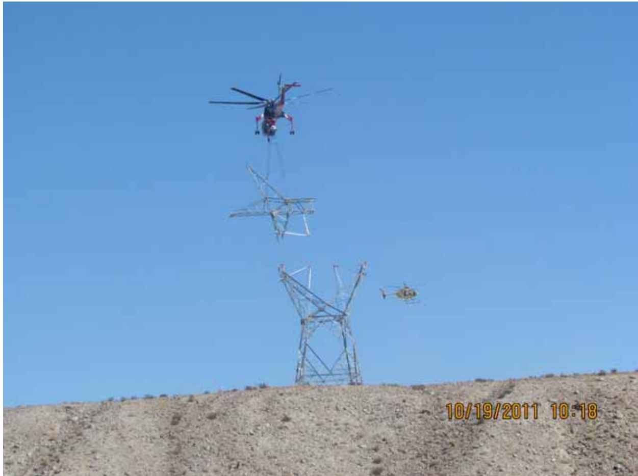
Erecting the 100 th lattice tower at EP290. Photo courtesy of Don Anders.
