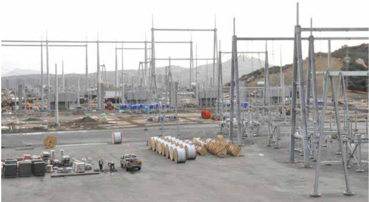
Suncrest Substation. Photo courtesy of Linda Collins.
