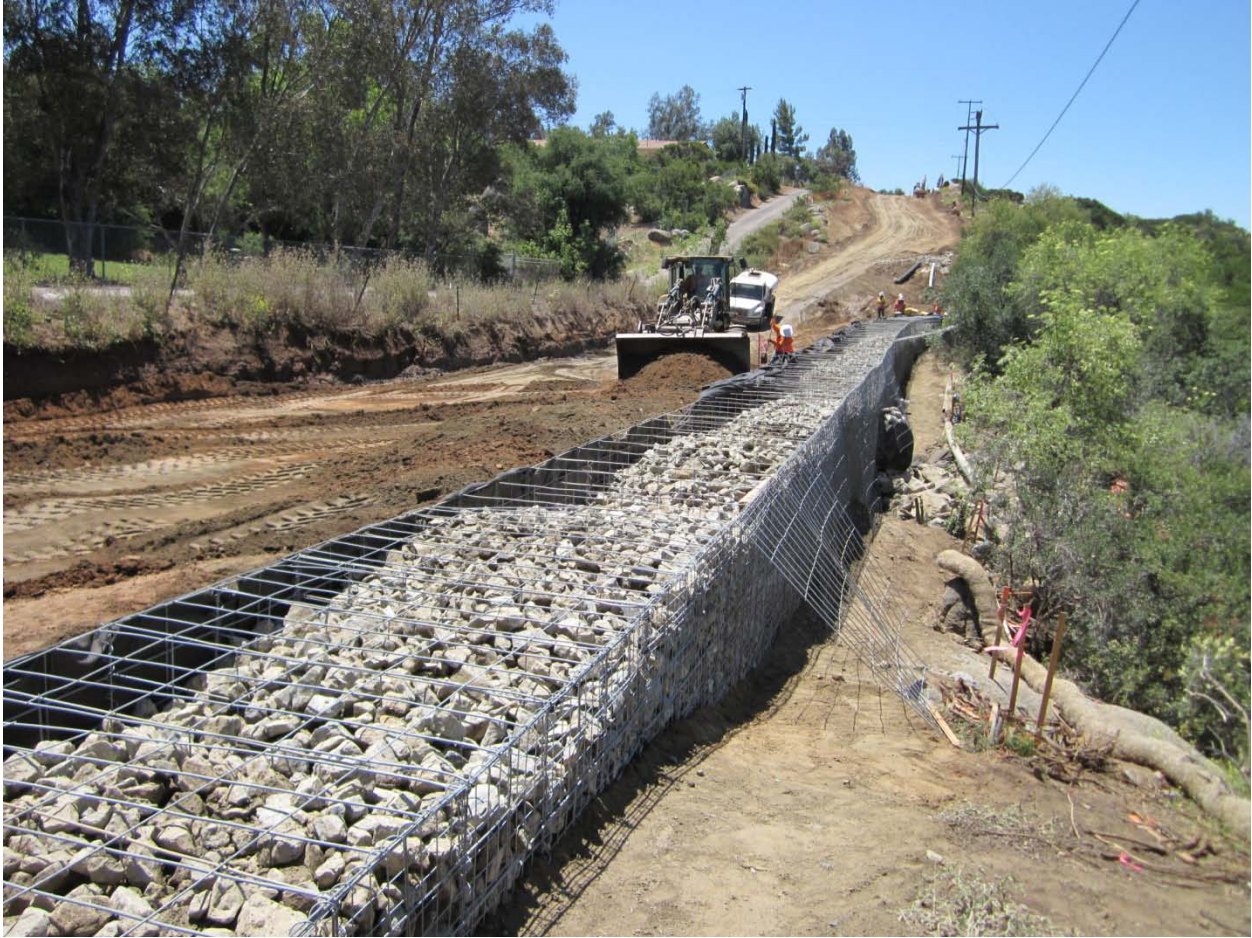
Loritz Property retaining wall. View to the south. Photo Courtesy of Jeff Smith.
