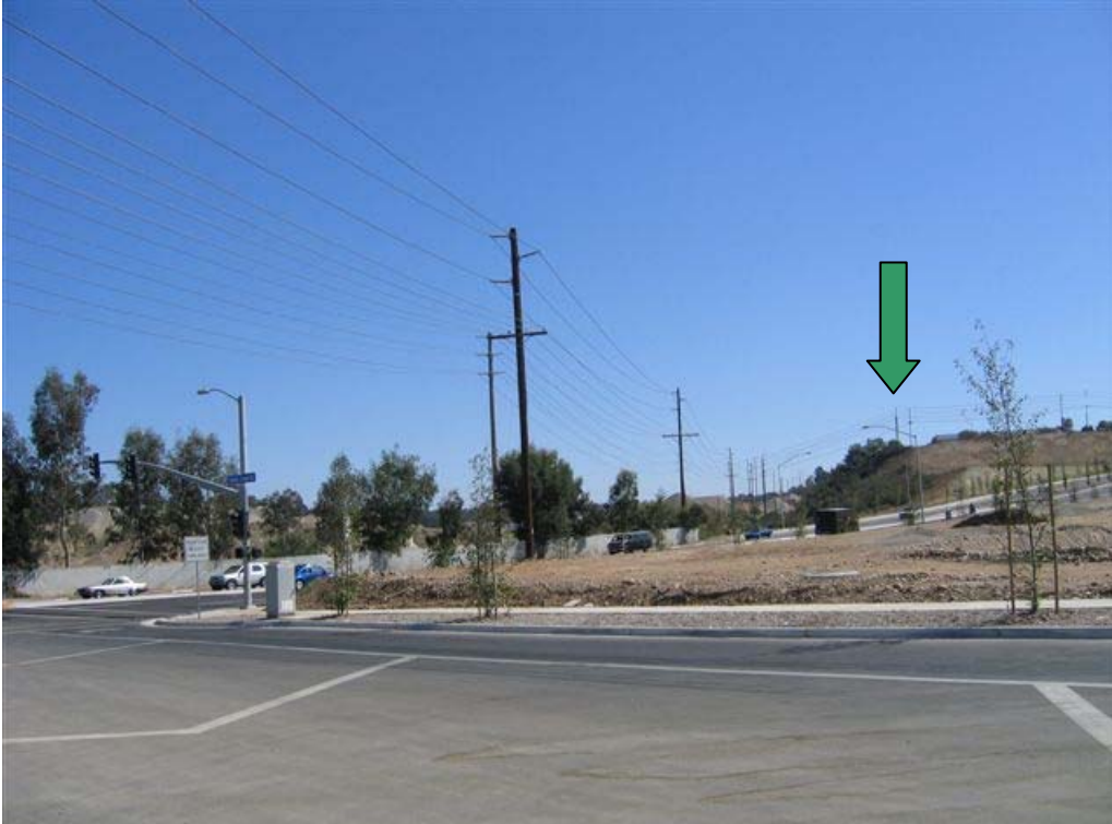
View of existing 69 kv lines through Fenton Canyon at the intersection of Camino Ruiz and Carroll Canyon Rd. Lines heading south to Miramar Substation are located just below green arrow.
