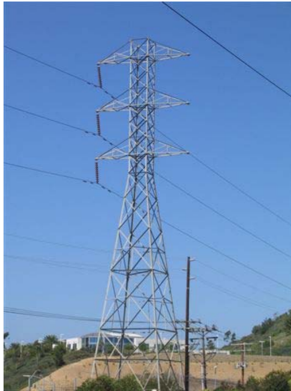
Vacant position on lattice tower located in SDG&E North-South ROW east of Interstate 805
