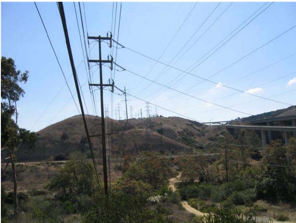
SDG&E North-South ROW east of Interstate 805 looking south
