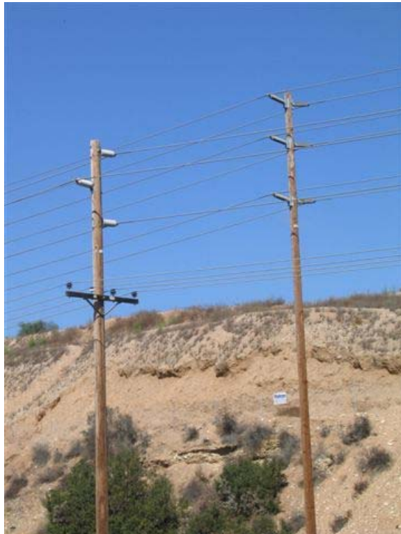
Closeup view of existing 69 kv lines through Fenton Canyon.
