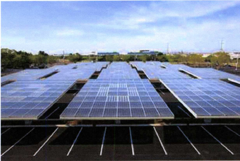
Photovoltaic parking lot
