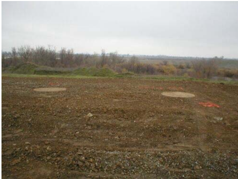
Figure 2 –Repaired sinkage problems at Vault locations along New Vineyard Road, Phase One.
