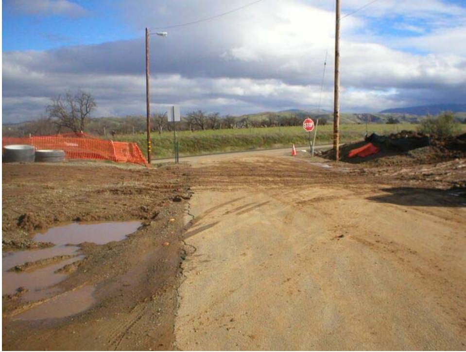
Figure 3 Dirt tracked into the road near the Vault 3A and 3B construction.
