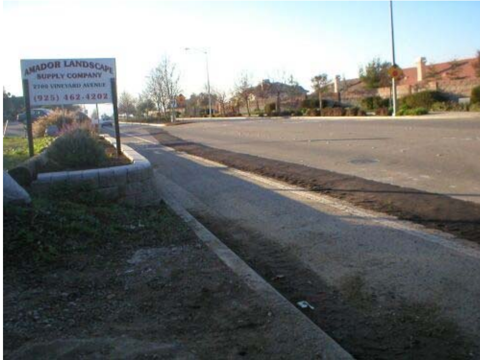
Figure 1 Temporary backfilled trench line within Vineyard Avenue to allow vehicle passage during non-construction hours.
