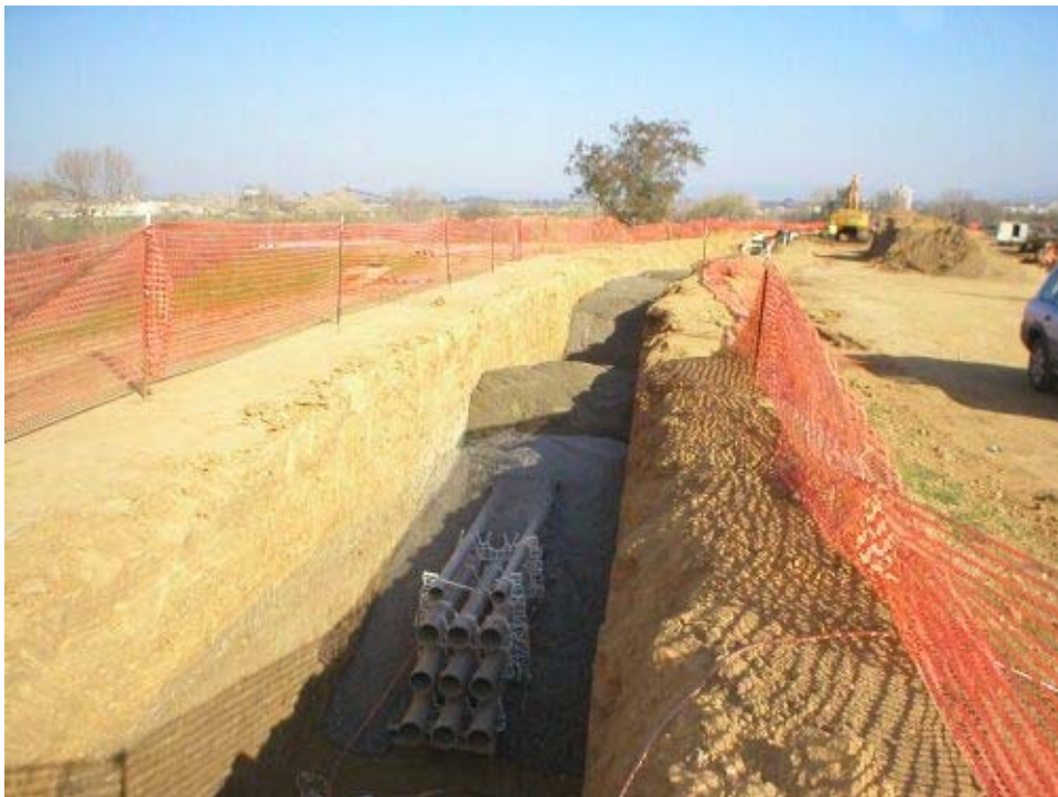
Figure 4 Conduit installation within trench along New Vineyard Road west of Vaults 14A and 14B.
