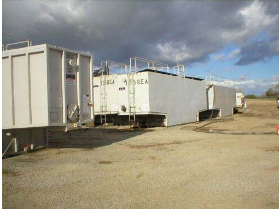
Figure 1 Arroyo del Valle northern bore pit. Overland discharge of contaminated water was prohibited by the RWQCB. Three 20,000-gallon Baker tanks were brought to the site to contain the groundwater.
