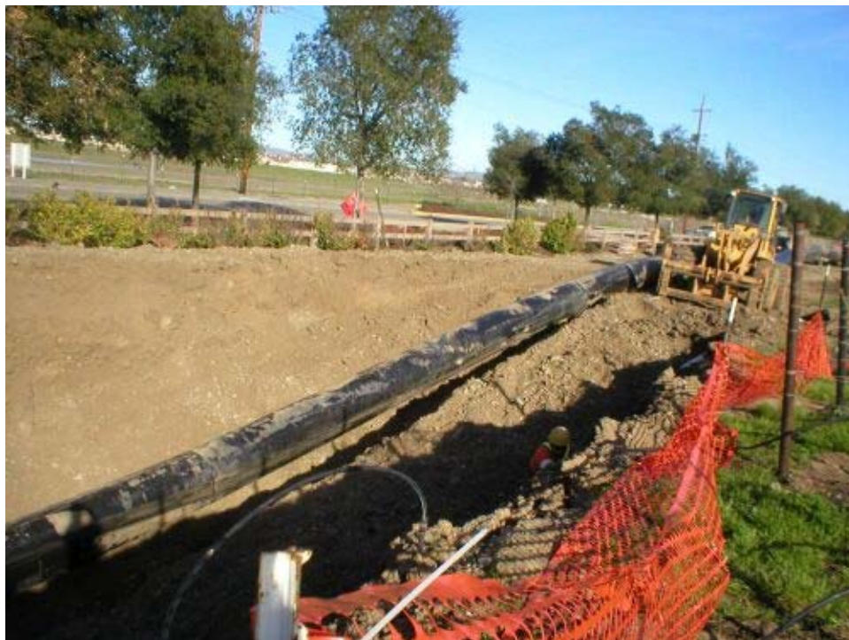
Figure 2 Ruby Hills, HDPE conduit welded for pull back through the bore hole.
