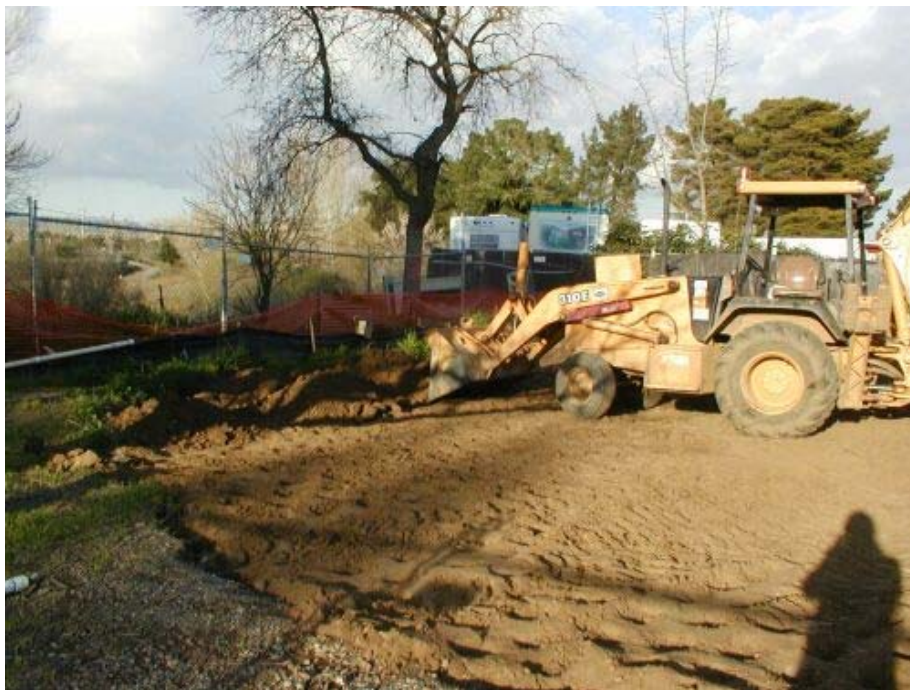
Figure 2 South Side of Arroyo del Valle Bore, the pit has been backfilled and compacted.
