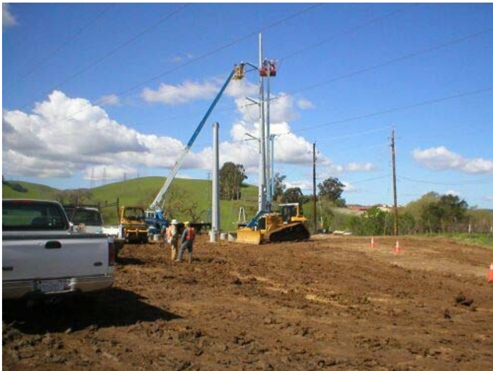
Figure 5 Transition Station, line-stringing operations to the erected pole structures. Note the lines were being grounded at the TEWS locations on both sides of the station.
