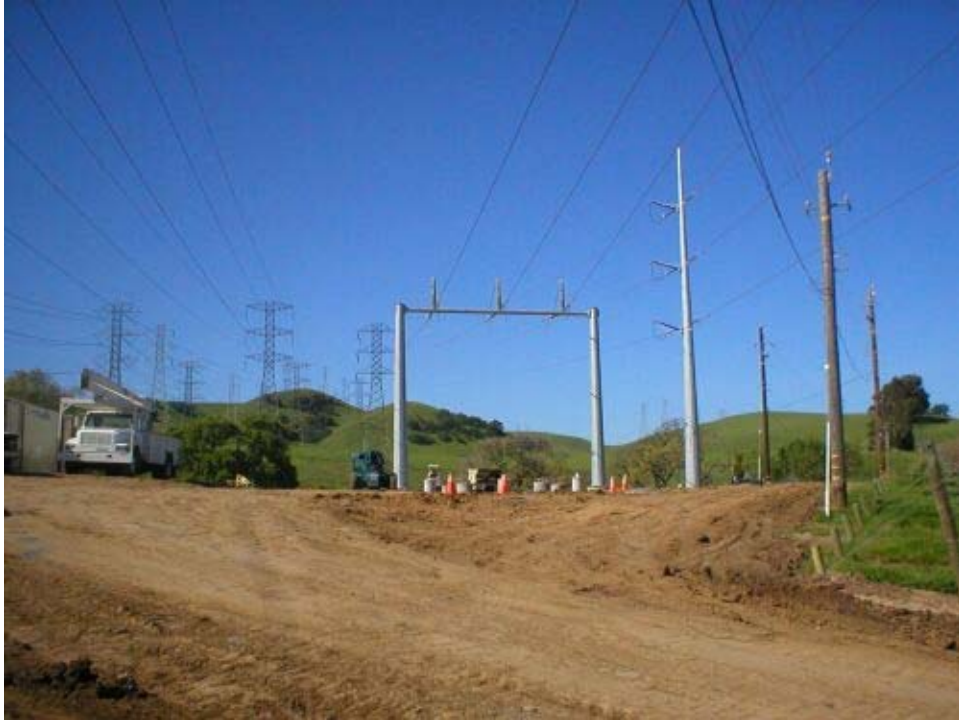
Figure 3 Transition Station Work. Note the new connections to the existing Contra Costa-Newark transmission line, which overhangs the Station area.
