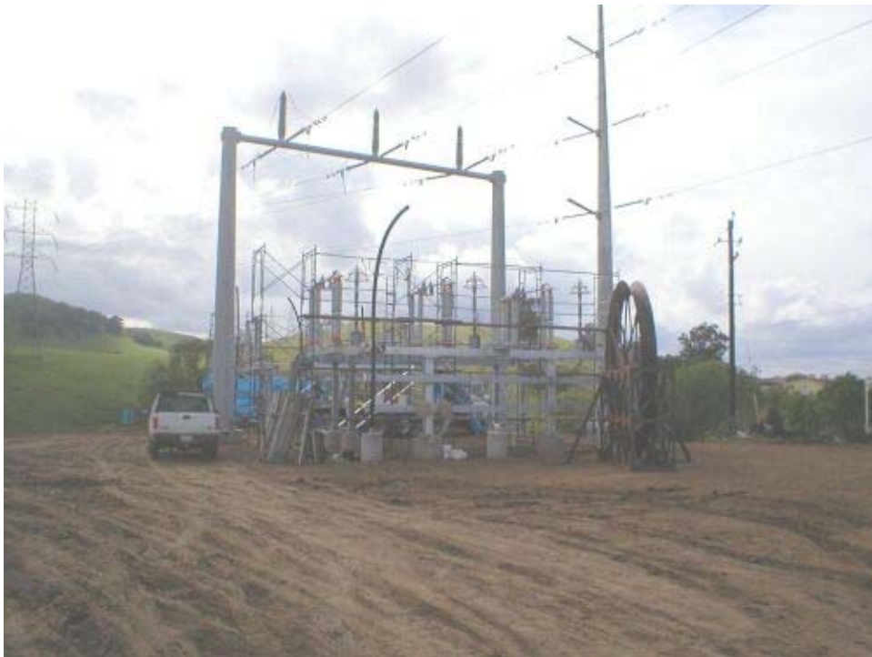
Figure 5 Continued work at the Transition Station, crews were on-site stringing conduit from the underground section to the above ground installation.
