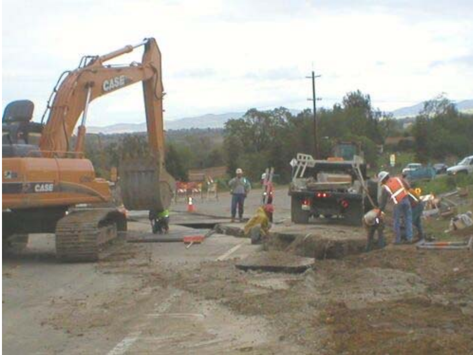
Figure 1 Trenching and conduit installation east of the Vault 15 location across “Old” Vineyard Avenue.
