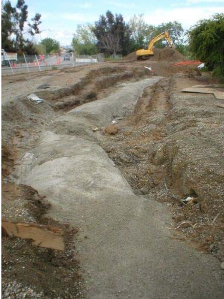
Figure 1 - Tie-in to south of the Arroyo del Valle. Concrete was poured over the conduit.
