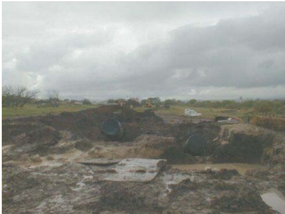
Figure 1 - New Vineyard Road Tributary Bore both HDPE casings have now been pulled back under the crossing.
